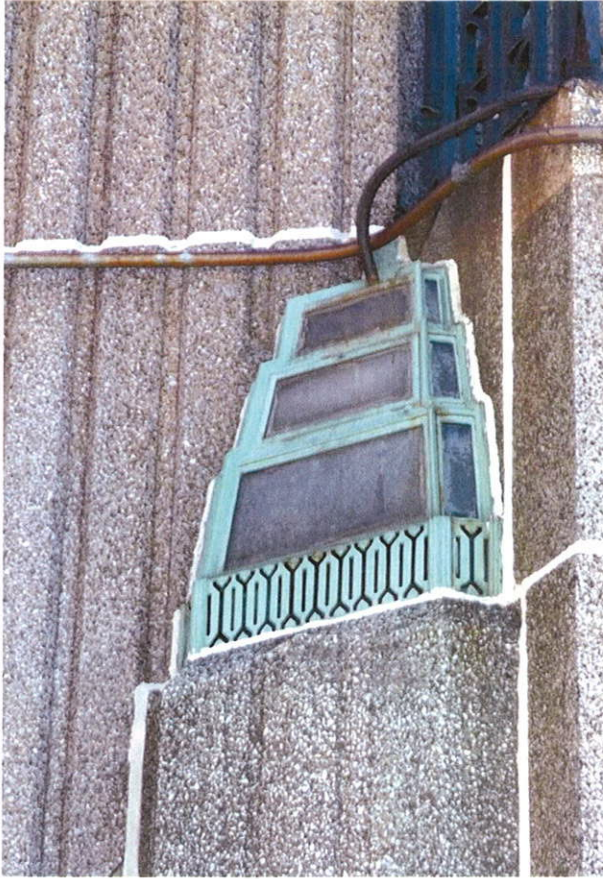
7. Entrance lamp detail.
