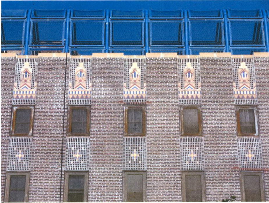
9. West façade detail with typical polychrome terra cotta at window heads and spandrels.
