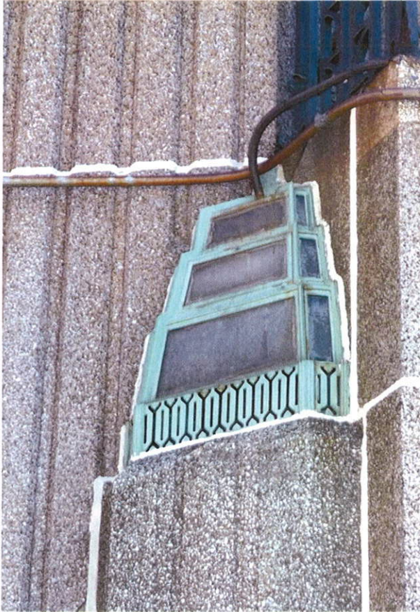
7. Entrance lamp detail.
