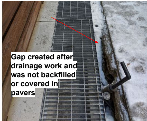
Damaged brick has been on a list of requested repairs since 2017
