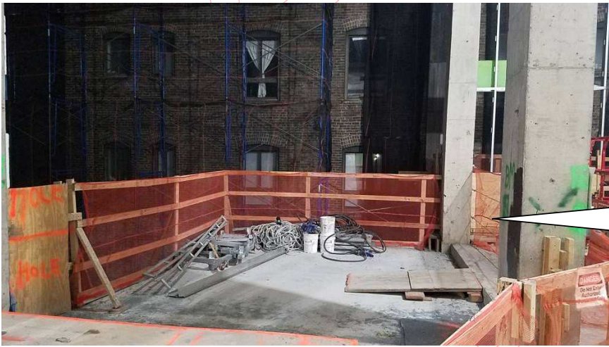
This is a view of the rear enclosed restaurant space on the 2 nd floor.
