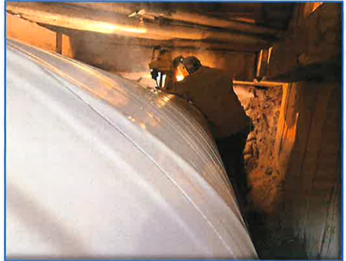
Welding the West 36" Trunk Water Main at 9 th Avenue and W.52 nd Street
