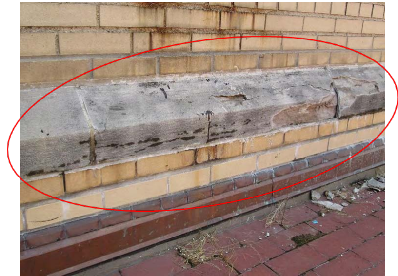
CRACK IN LIMESTONE LEDGE
