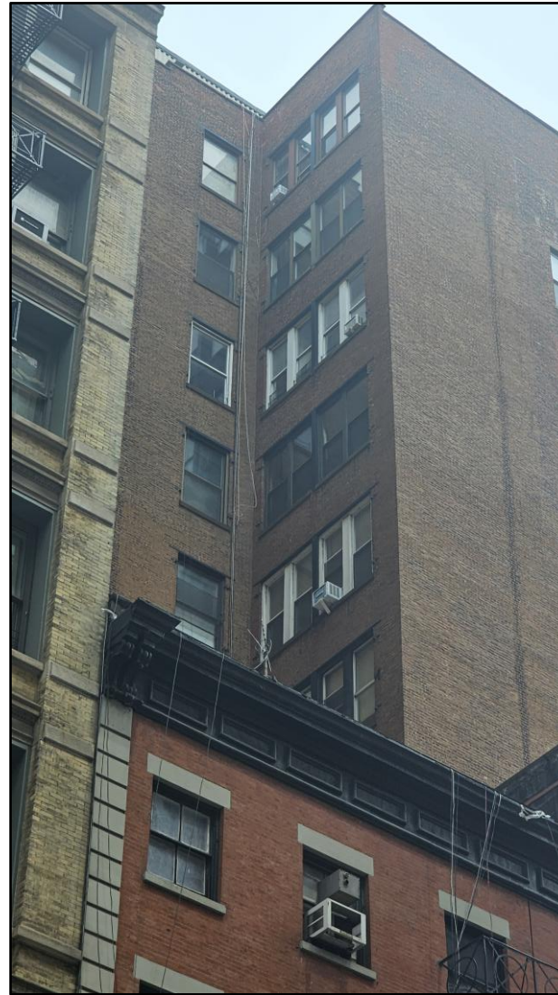
Previous windows at west lot line return wall, zoomed in. Summer 2025. (Metamechanics)
