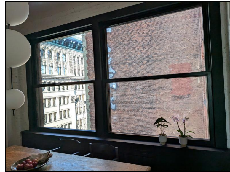
Windows replaced at west lot line return wall, seen from the interior. April 2026. (J. Peu-Duvallon)
