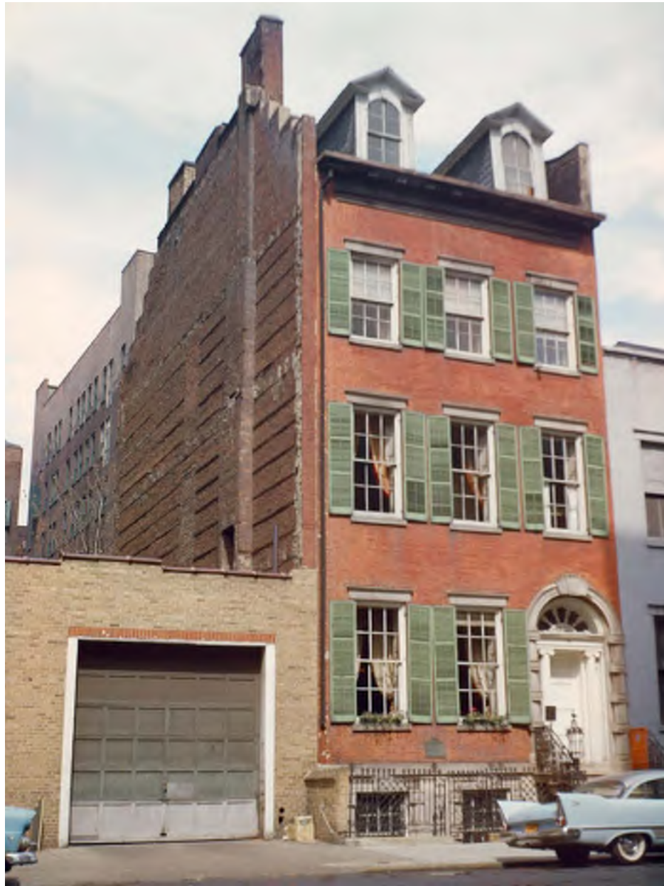
1960'S LOT LINE WALL CONDITION
