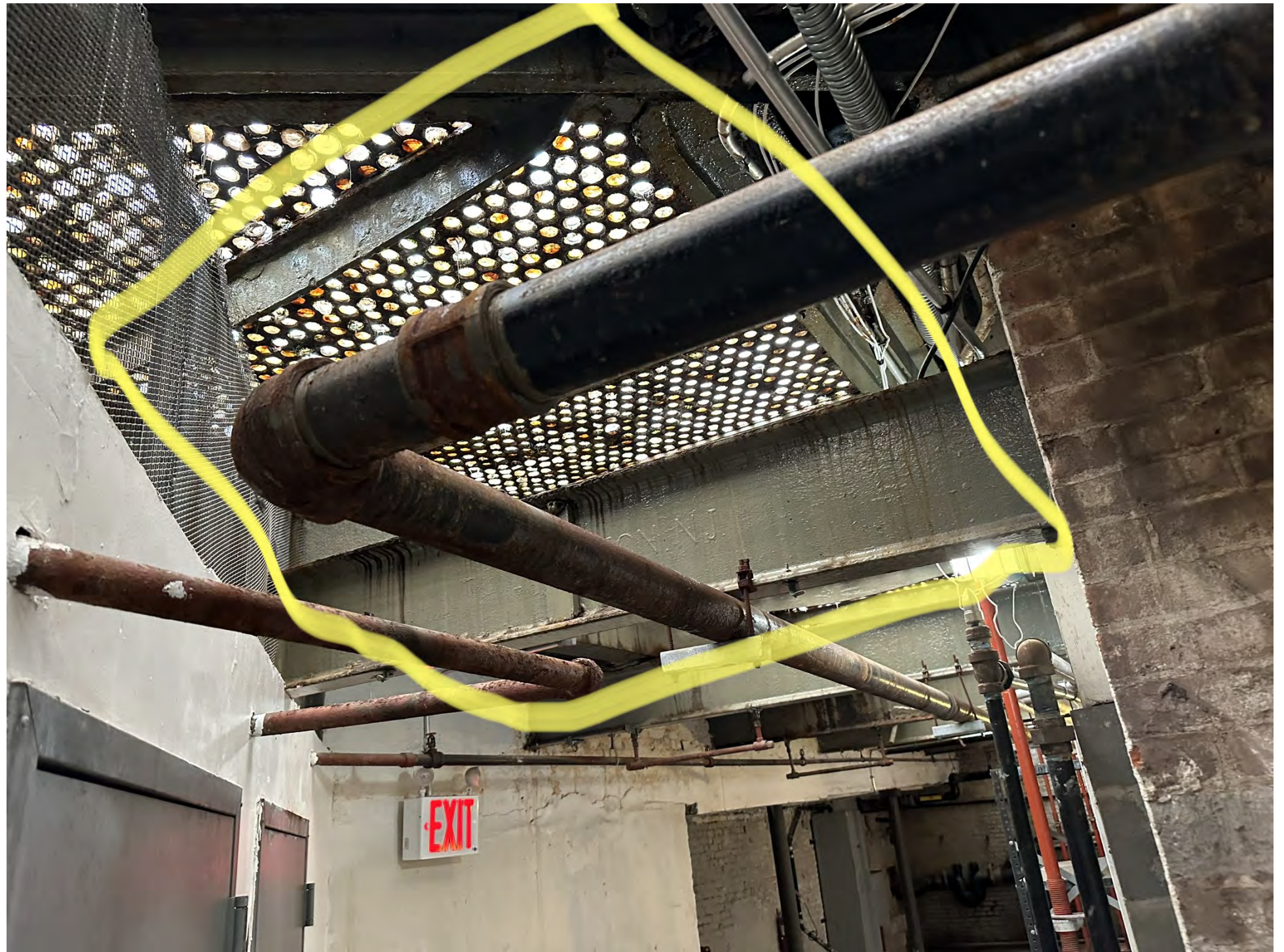
22 BASEMENT DAMAGE Scale: NTS
