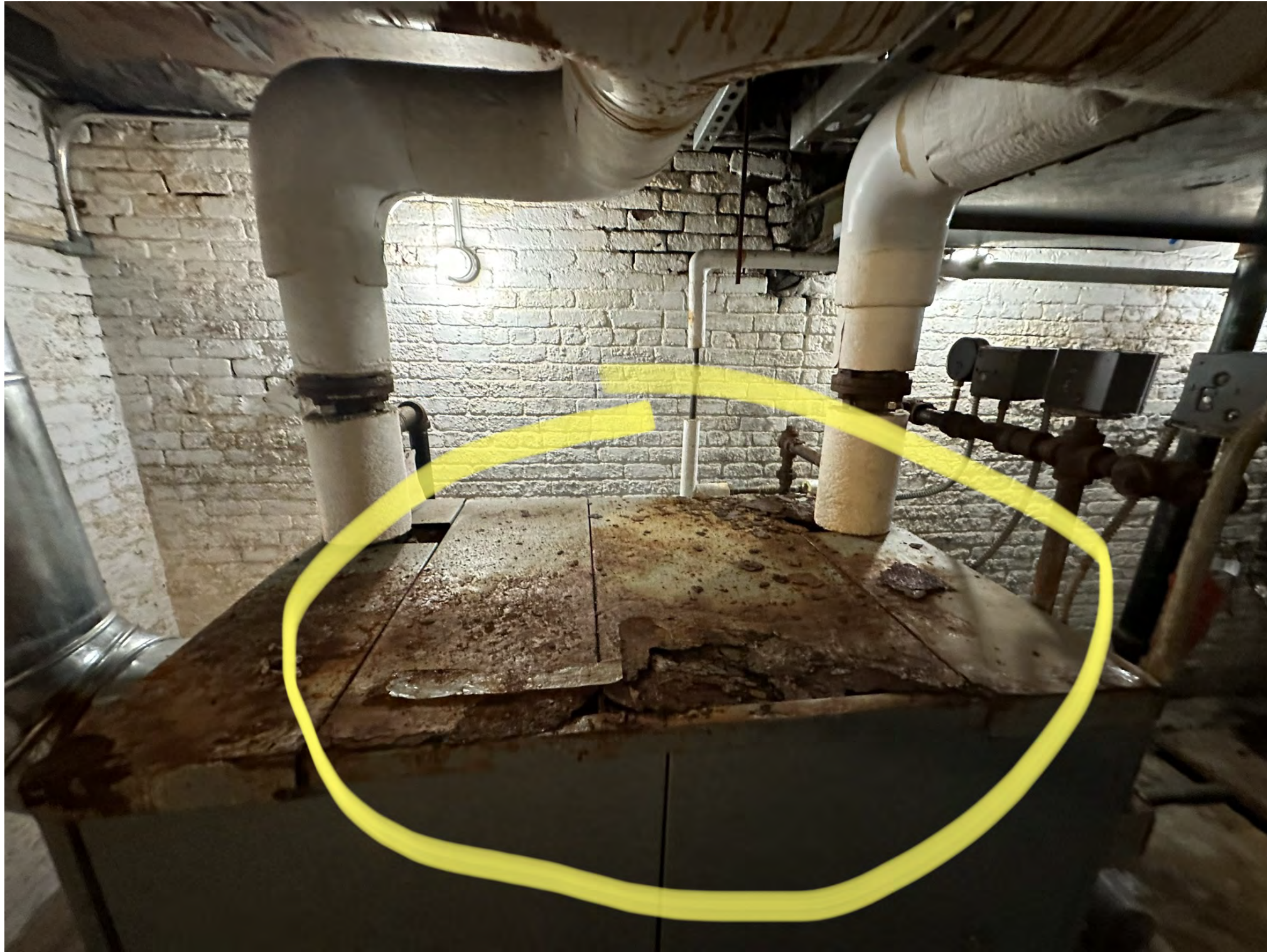
23 BASEMENT DAMAGE @ BOILER Scale: NTS
