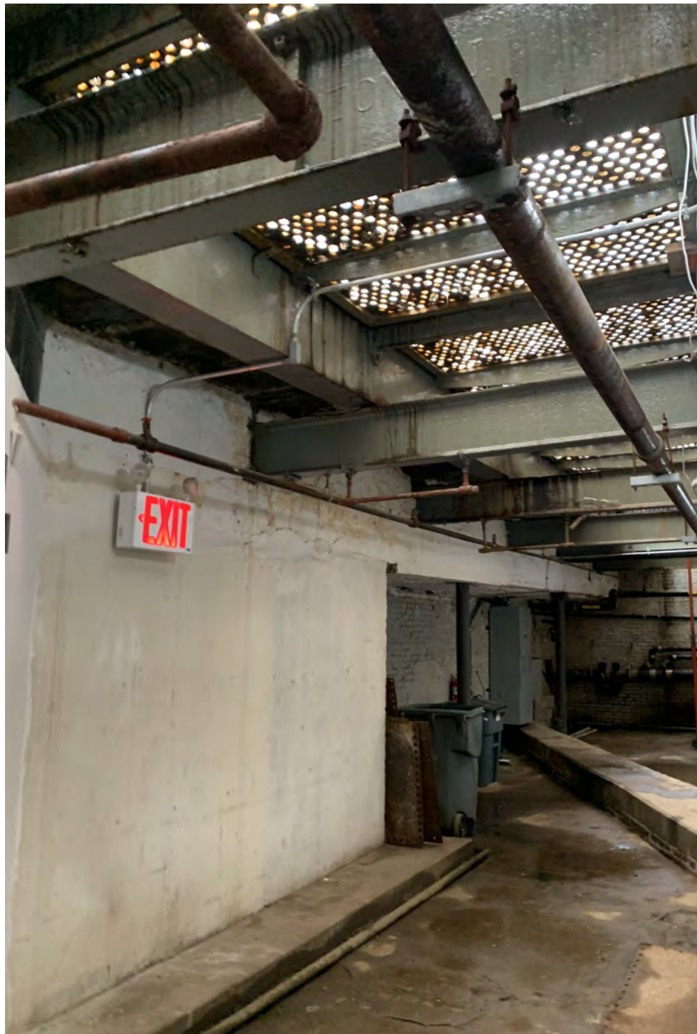
21 BASEMENT DAMAGE Scale: NTS
