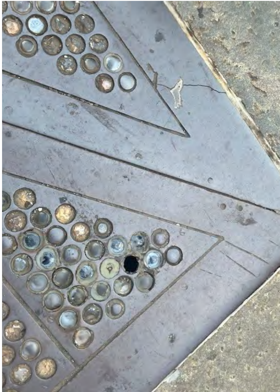
09 Damaged Frame and Glass Close-Ups Scale: NTS
