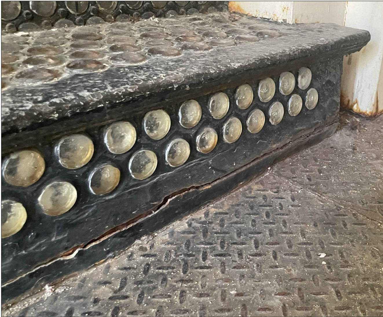
SOUTH STEPS (DAMAGE AS SEEN FROM ABOVE)
