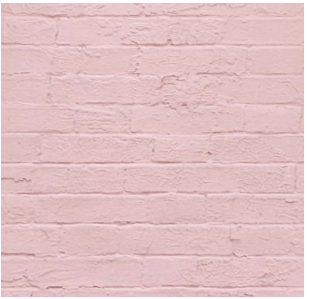
Existing pink painted brick to be restored
