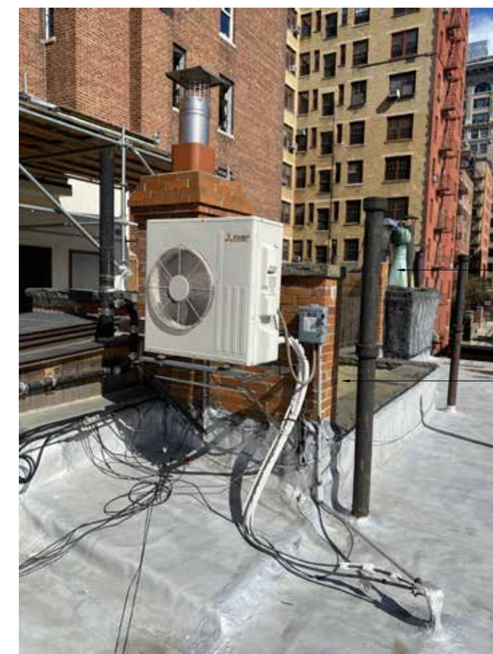
1 SITE PHOTOS: EXISTING AC UNIT NTS
