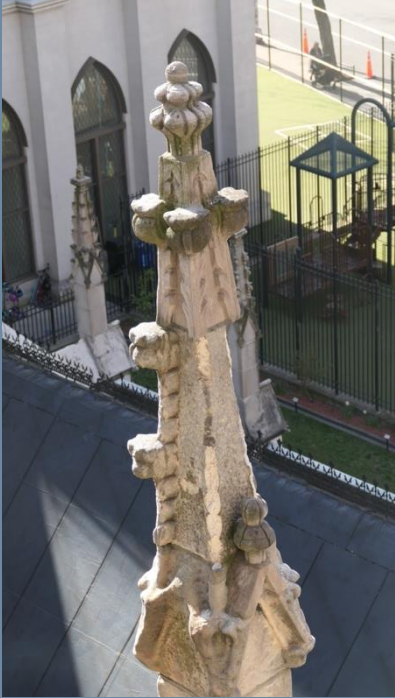
Cracked and spalling decorative units.
