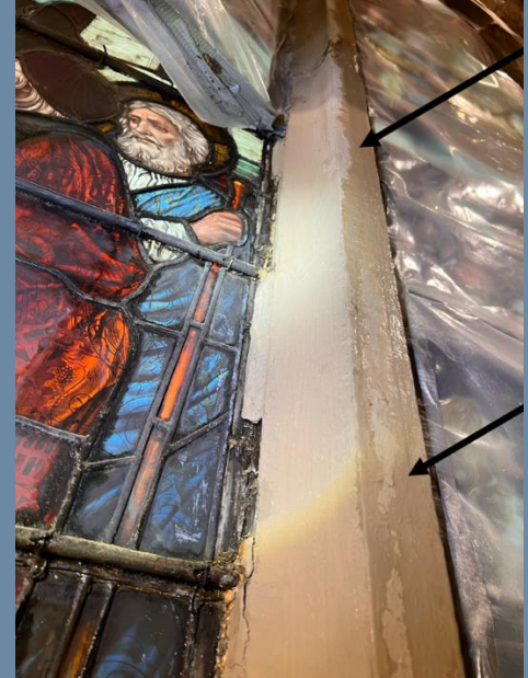
Interior water infiltration.
