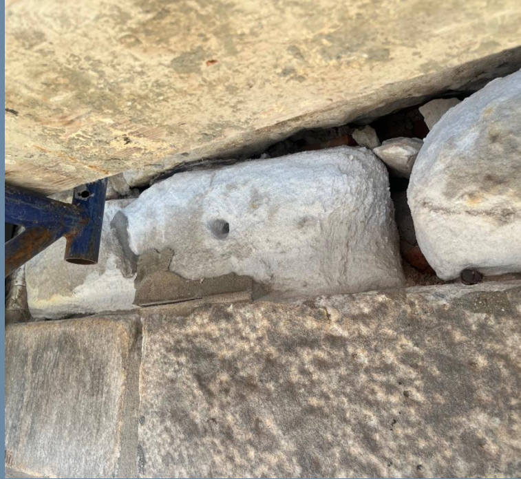
Eroded and missing ashlar stone units.
