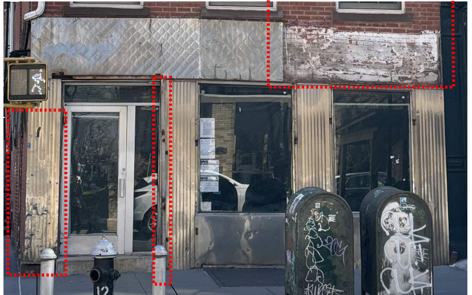
Stainless steel cladding severely dented, with exposed fasteners and missing base trim in potentially hazardous condition
