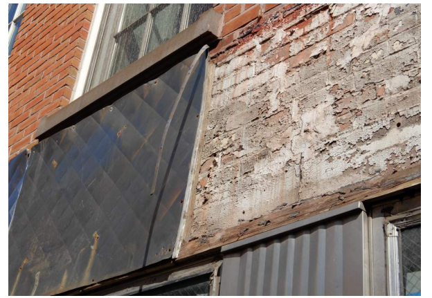
Stainless steel sign band in poor condition with missing panels
