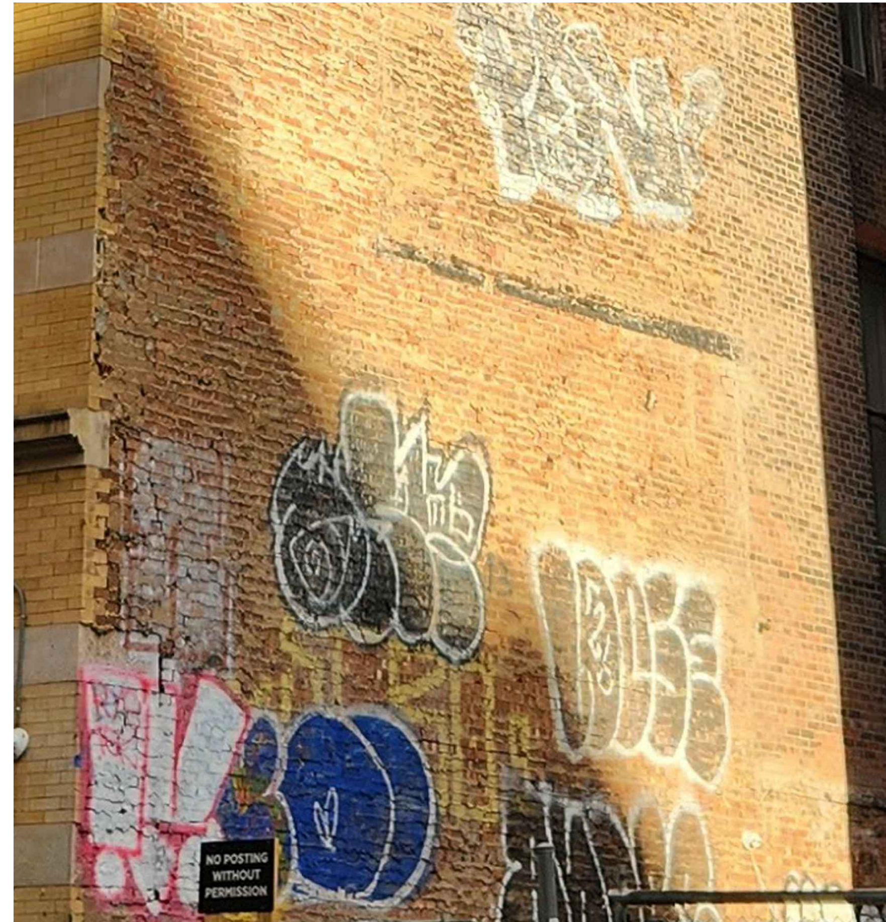
2 SOUTH ELEVATION, GRAFFITI AND OPEN JOINTS
