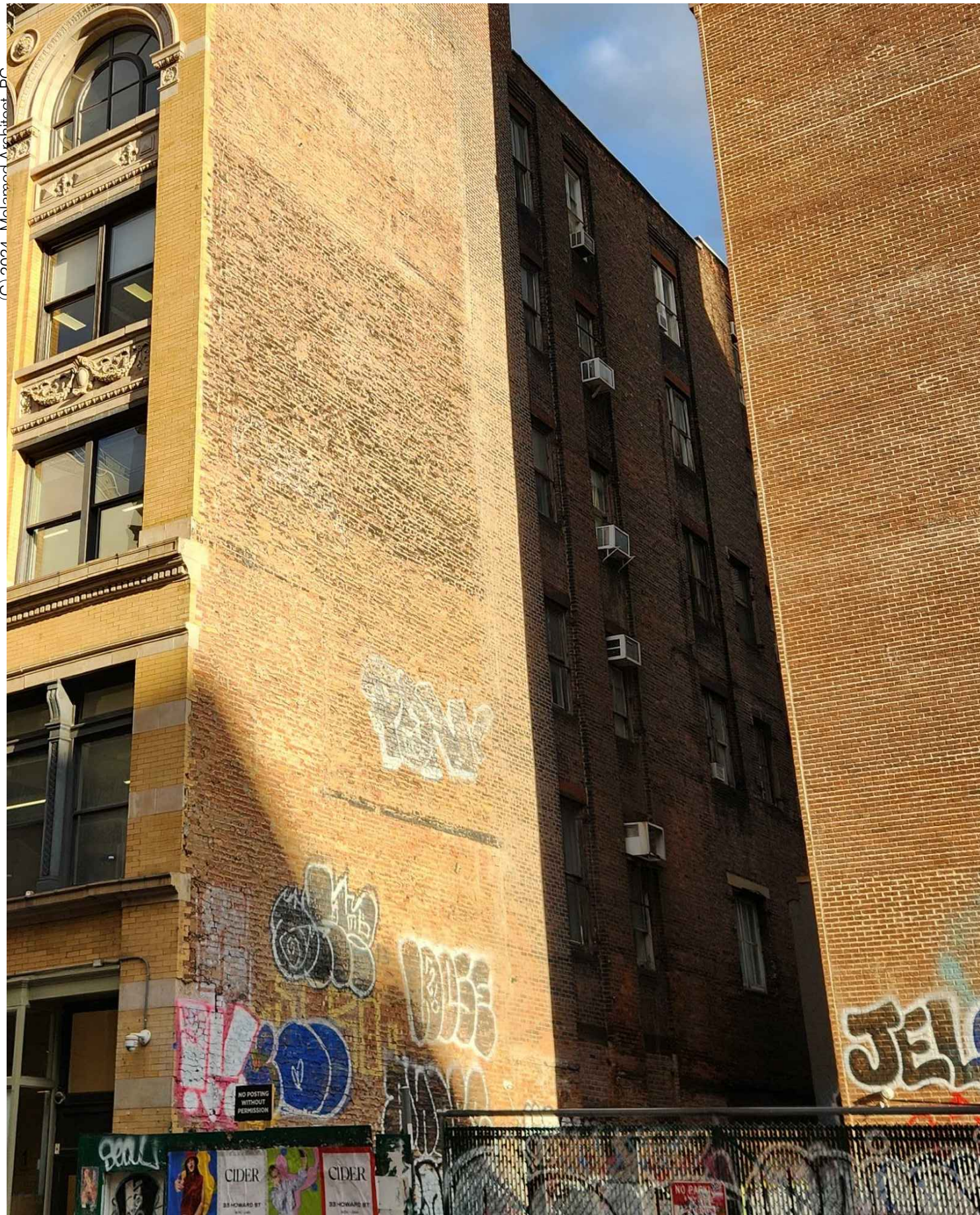
1 SOUTH ELEVATION, GRAFFITI & OPEN JOINTS
