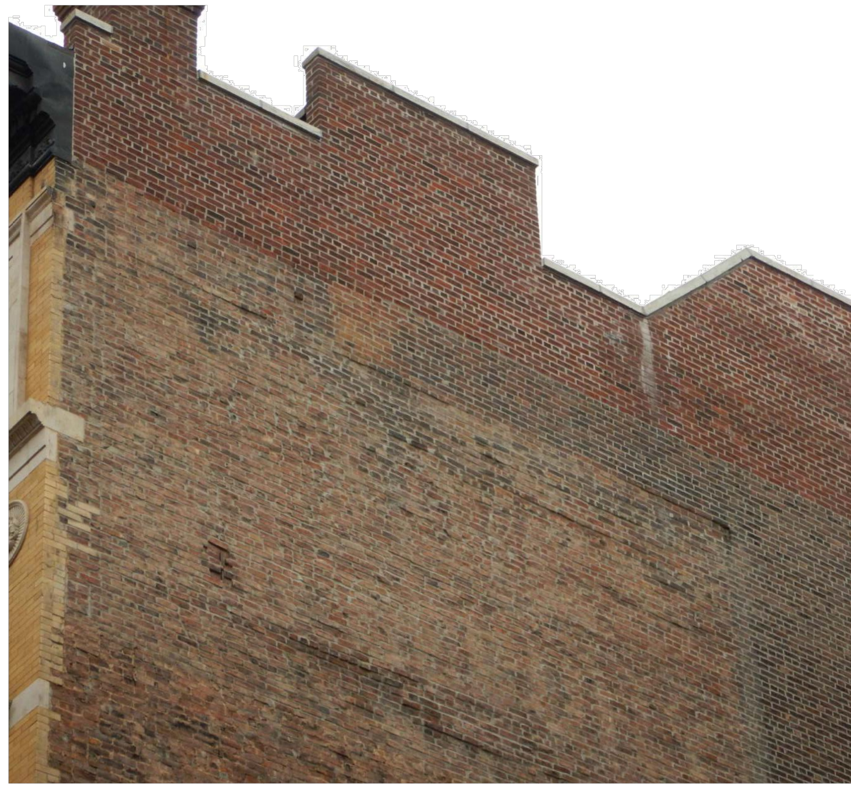
5 SW CORNER OF BUILDING, OPEN JOINTS & PREVIOUS REPAIRS
