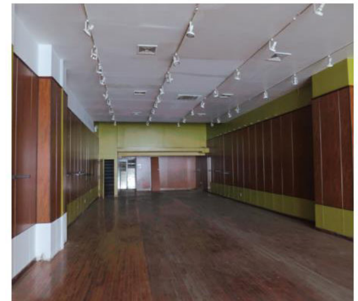
GROUND FLOOR. ORIGINAL REAR WALL IS NOT EXTANT AT GROUND FLOOR. IT WAS LIKELY LOCATED WHERE THE SIDE WALLS PROJECT OUT SLIGHTLY.
