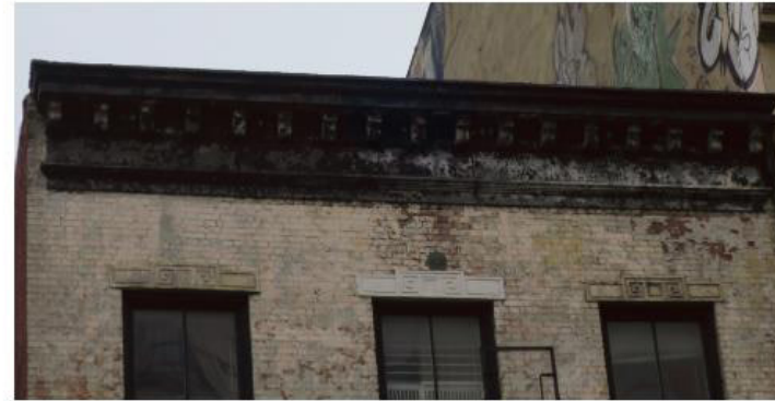
423 BROADWAY ITALIANATE SHEET METAL CORNICE. THE CENTRAL LINTEL AT THE TOP FLOOR APPEARS TO BE PARSED
