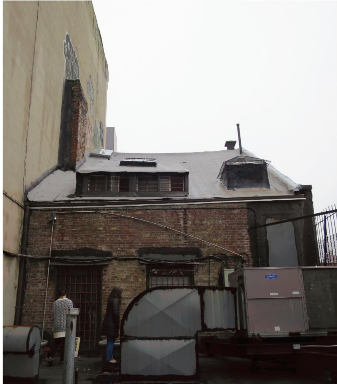
REAR ELEVATION. THE FACADE HAS COMMON BOND BRICK WITH SEGMENTAL ARCH LINTELS. THE ROOF IS CLAD IN A NON-HISTORIC ASPHALTIC MEMBRANE AND THERE ARE NON-HISTORIC DORMERS.
