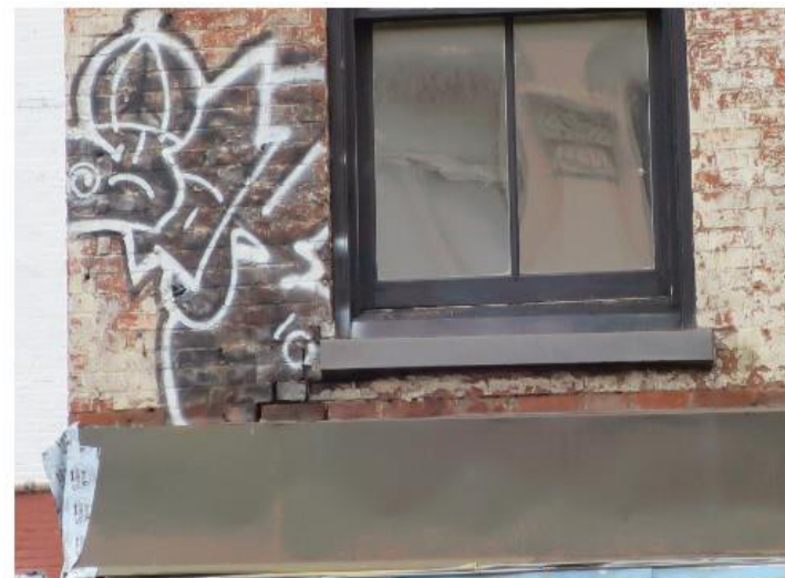
BROWNSTONE WINDOW SILLS HAVE NON-HISTORIC ALUMINUM CAPS. THE BRICK FACADE IS EXPERIENCING SOME STEP CRACKING. GRAFFITI EXISTS AT THE SECOND FLOOR OF THE PRIMARY FACADE AND ALONG THE SOUTHERN SIDE WALL.
