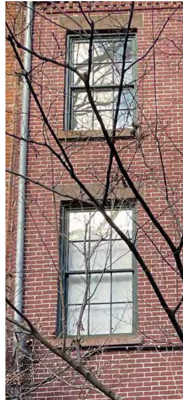
LEVEL 2 & LEVEL 3 WINDOWS
