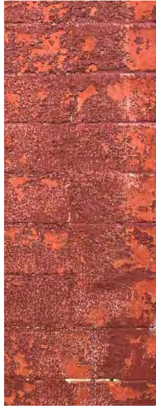
ORIGINAL BRICK VISIBLE BELOW PEELING PAINT
