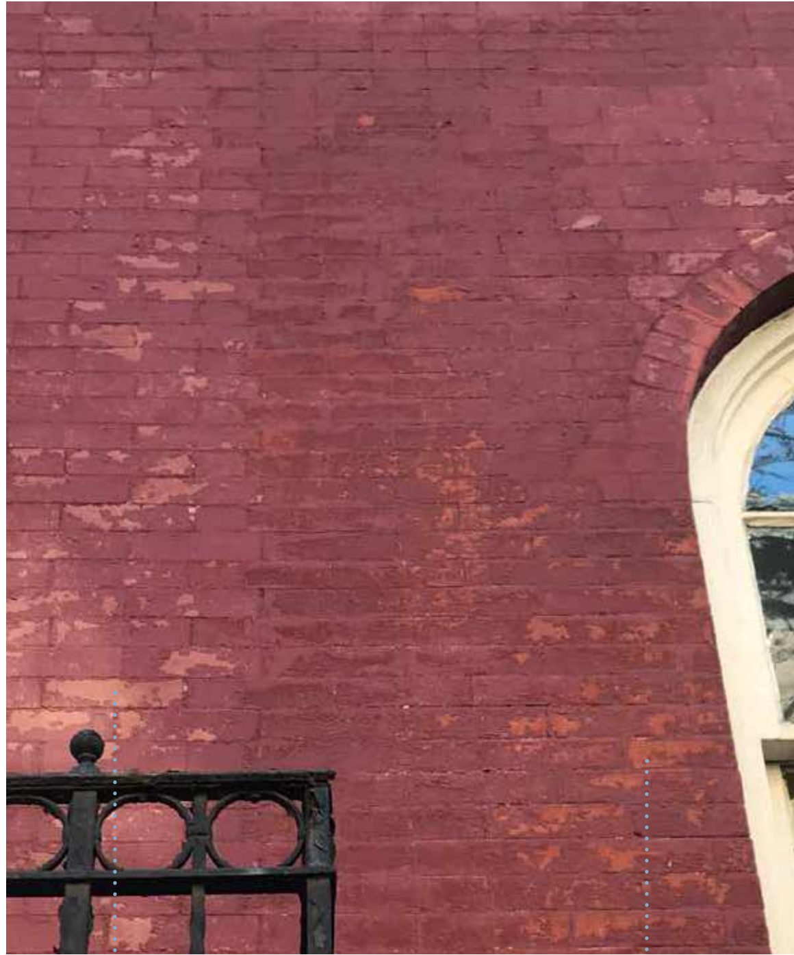
INFILL BRICK FROM 1924 CONVERSION VISIBLE BELOW PEELING PAINT
