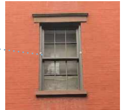
CAST STONE LINTELS AND SILLS TO MATCH 278 WEST 11TH STREET. LIGHT PAINTED DOUBLE HUNG WINDOWS (PROPOSED WINDOW COLOR NOT SHOWN ABOVE).
