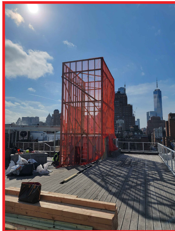
7* VIEW OF PASSENGER ELEVATOR FROM WEST SIDE
