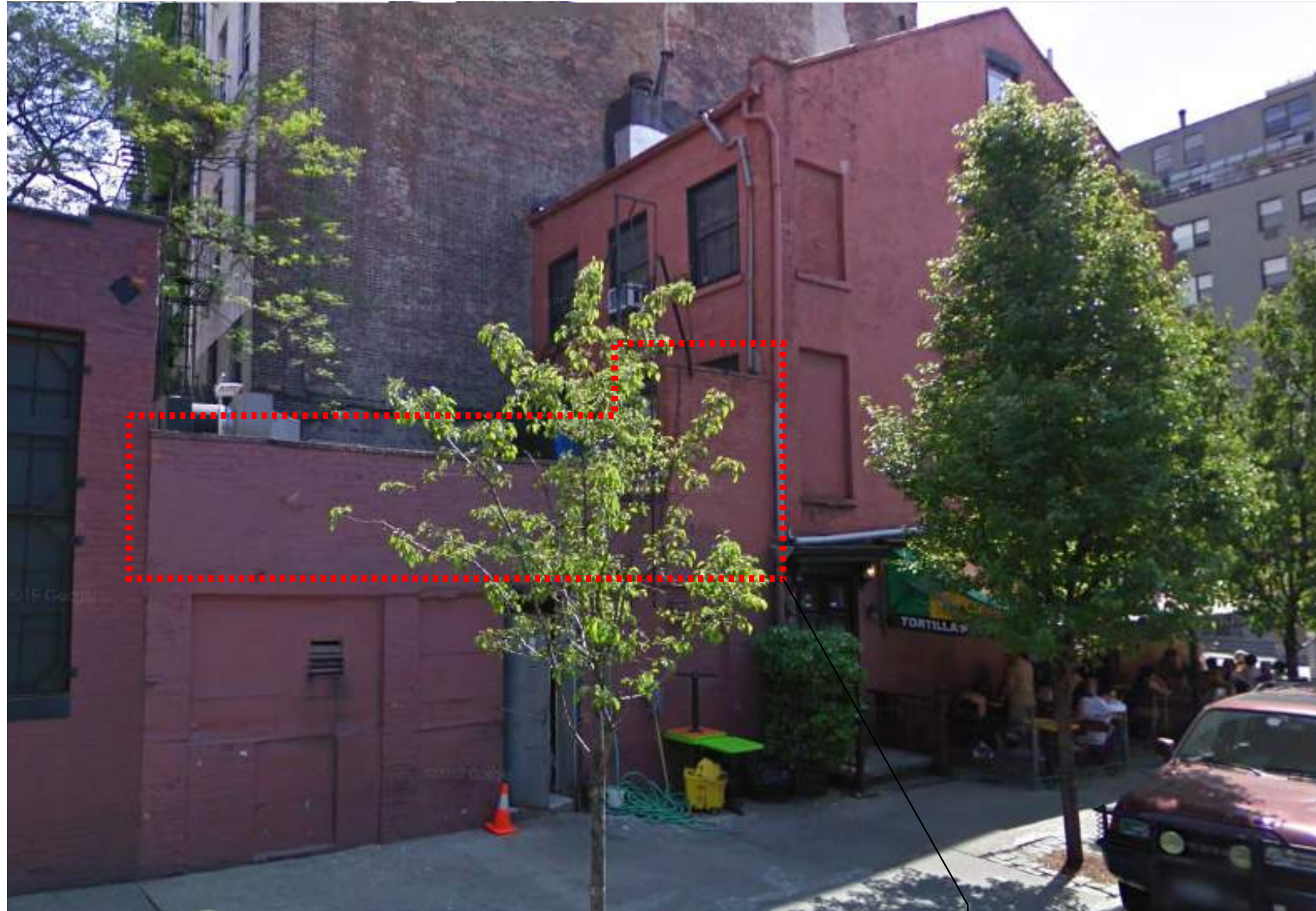
Coping, parapet and stone lintel removed under Alt-2 121090283, refer to drawings and LPC application for clarification of scope
