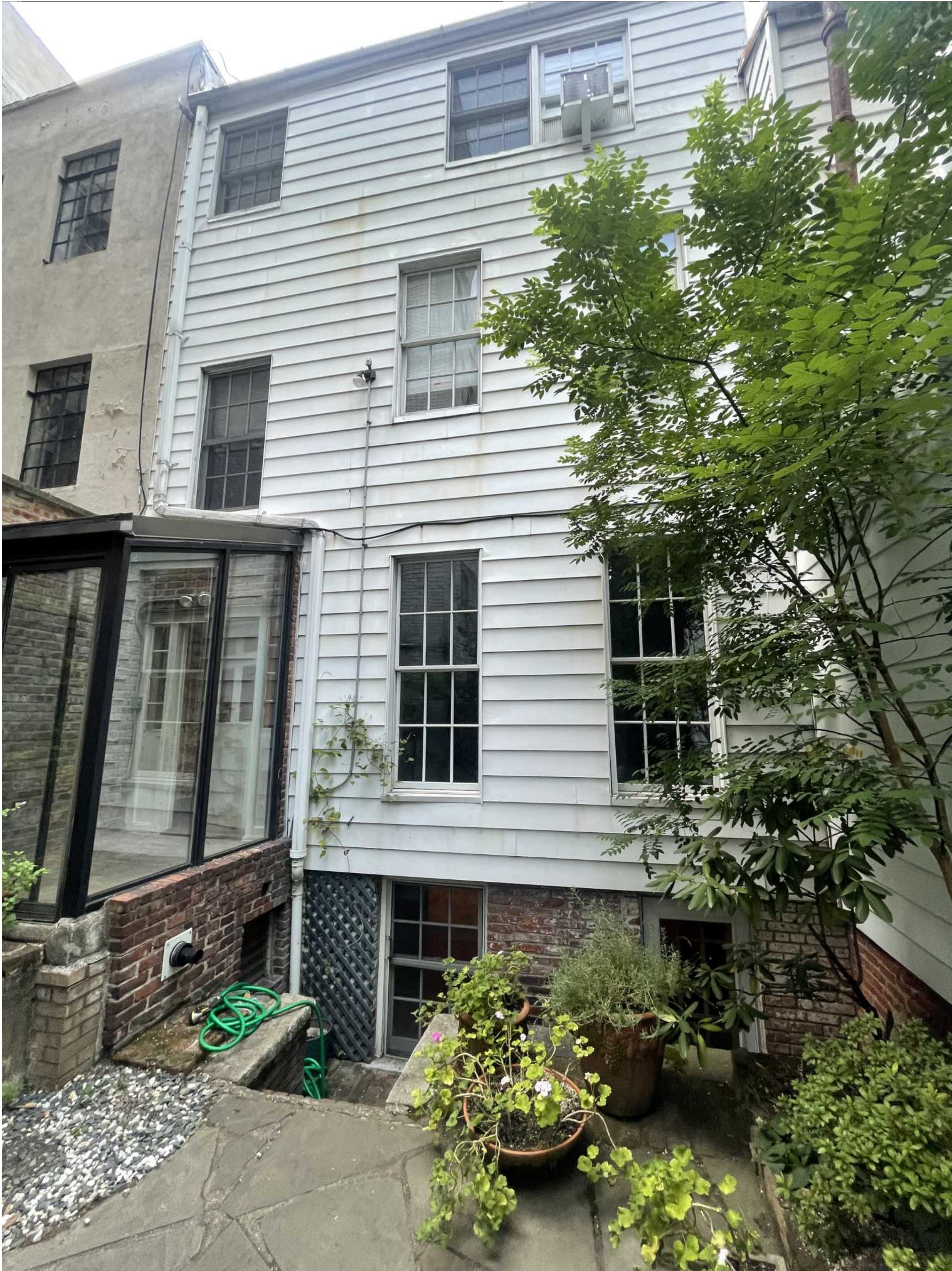
4 grove street rear facade c. 2023
