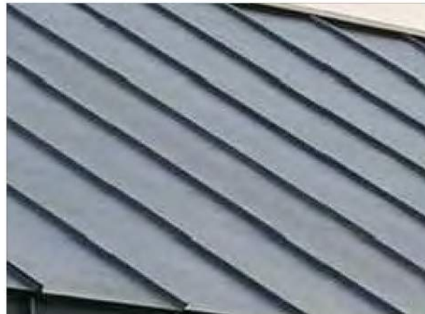
3 4TH FLOOR PITCHED ROOF - ZINC COATED DOUBLE STANDING SEAM LPC-152.00 SCALE: NTS
