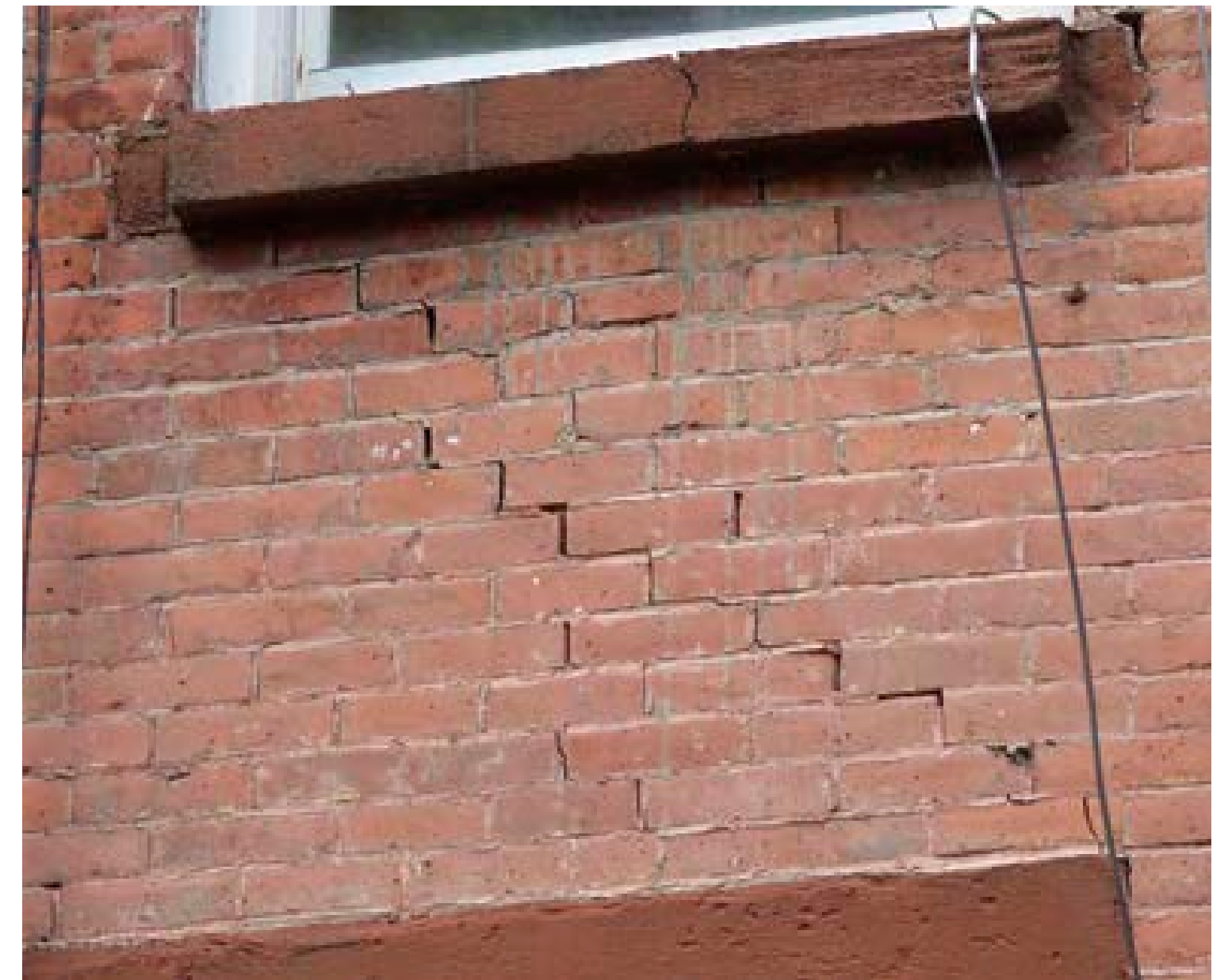
Detail of the brick between the parlor and second floors, showing step cracking and a crack through the stone sill
