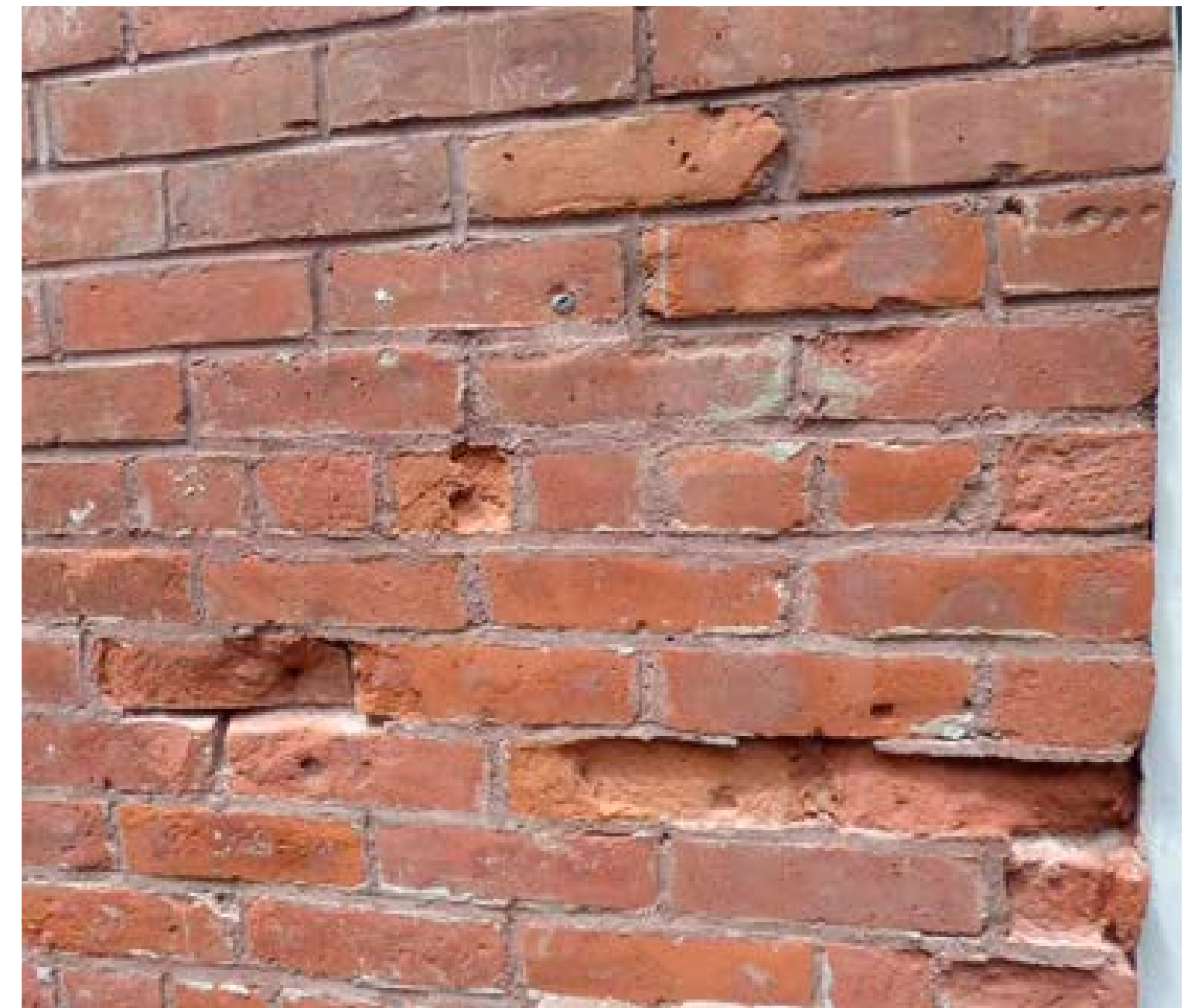
Detail of the brick at the ground floor, showing lack of a fire skin and significant spalling
