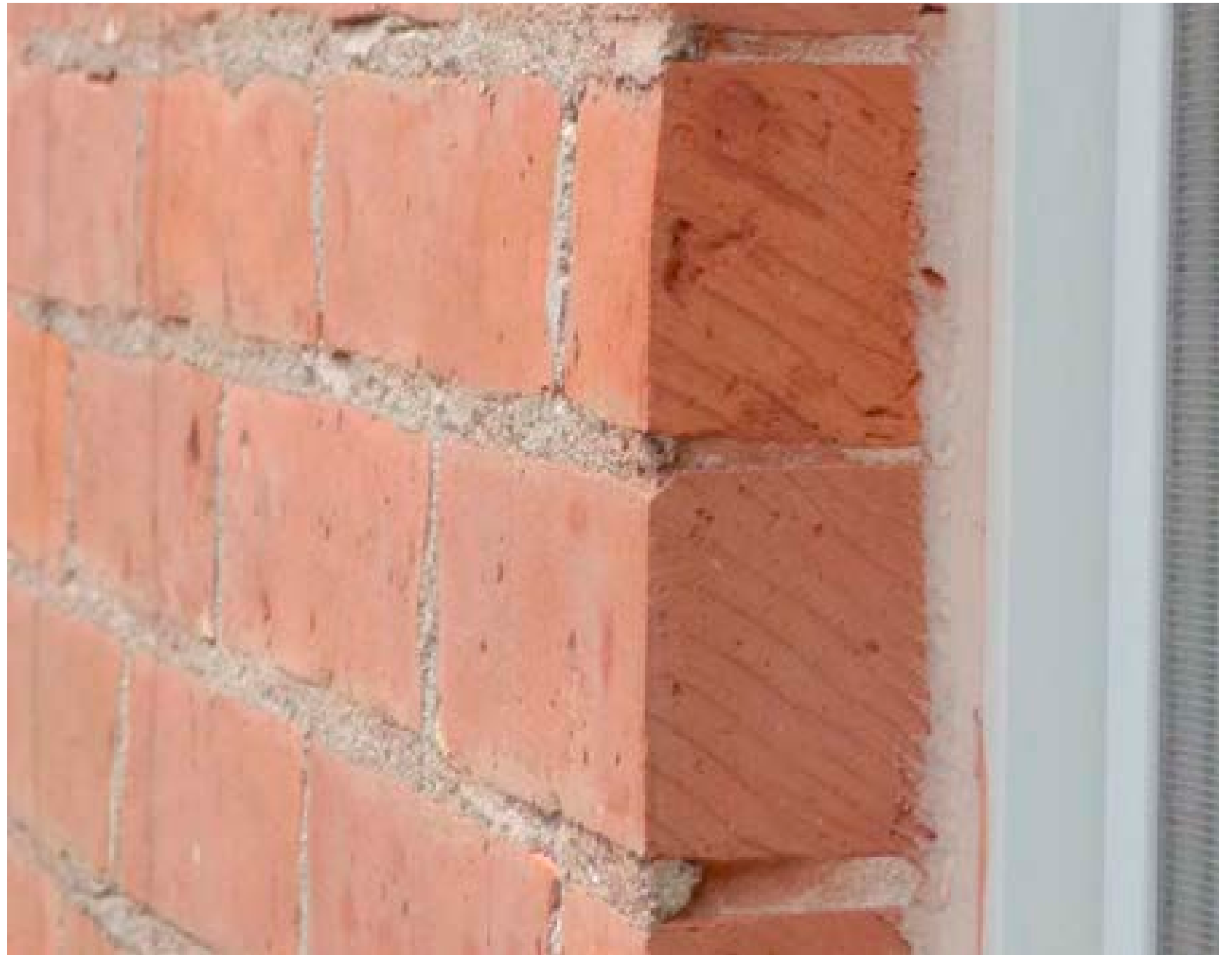
Detail at Parlor Window, showing visible circular abrasions
