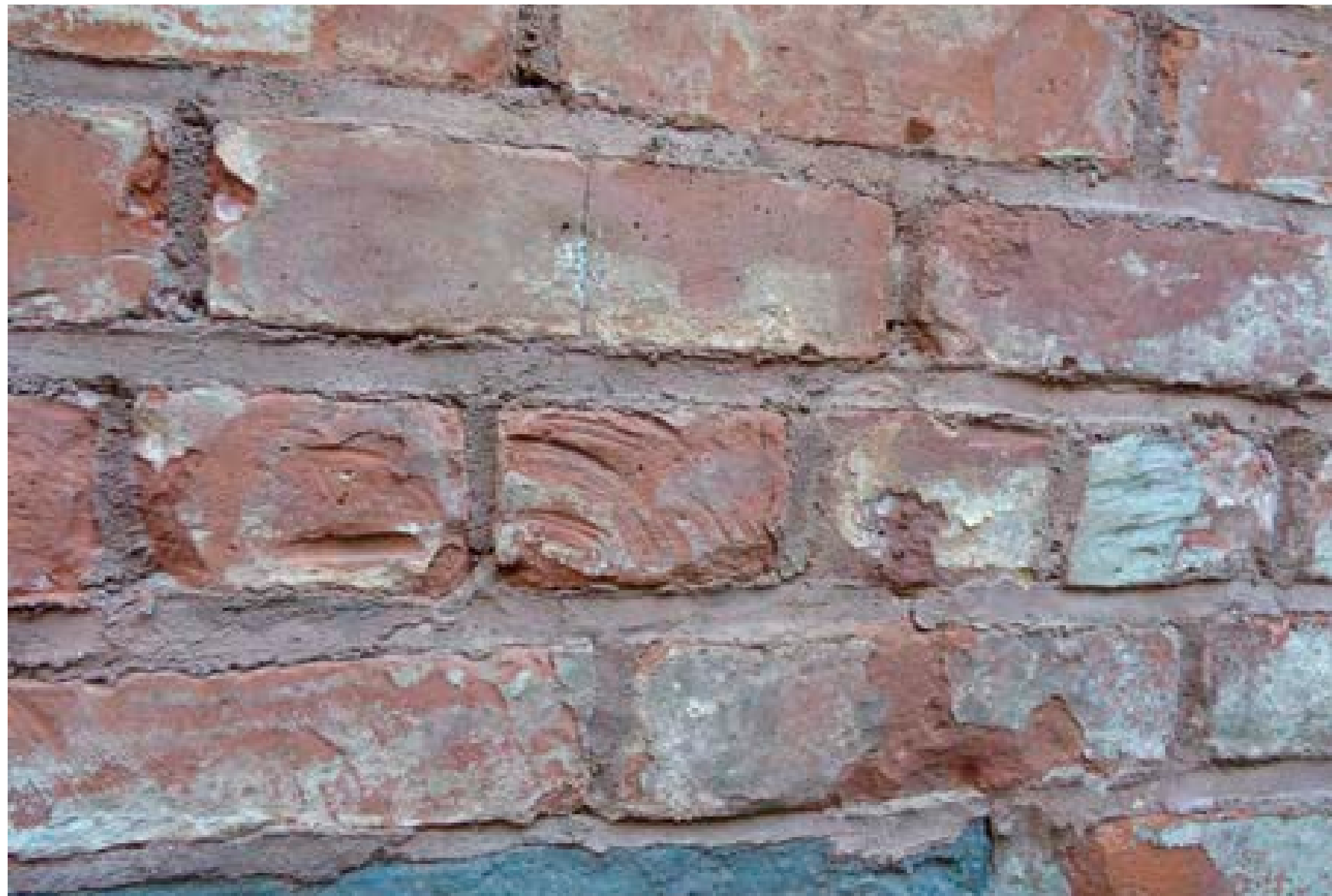
Detail of brick at the rear facade showing typical conditions, including abrasions from a mechanical grinder, spalling and material loss, efflorescence, and improper mortar type.
