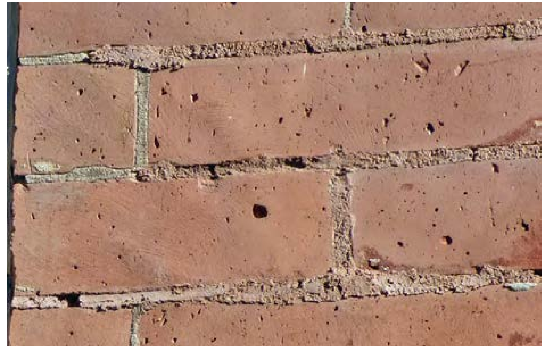
Typical conditions, including visible abrasions and loss of the fire skin
