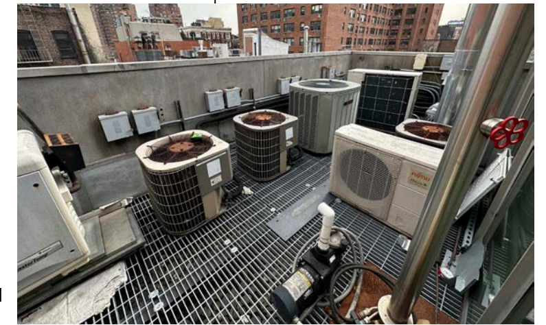
Existing mechanical equipment
