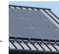
Metal structure for solar array
