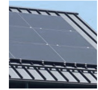
Metal structure for solar array
