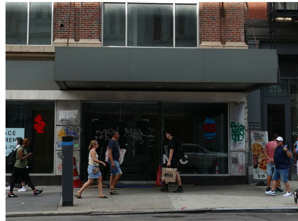
Original terra-cotta piers at the base have been removed or covered up; existing historic fabric that can be maintained will be repaired and missing piers will be recreated. The existing marquee structure will be reclad.
