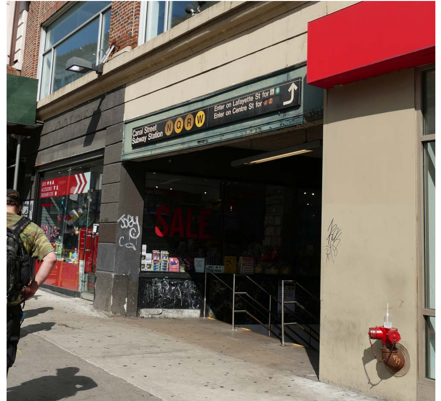
There is a subway entrance at Broadway with non-historic storefront infill at its interior walls. A cementitious coating has been applied to the extant terra-cotta piers at this area of the building.
