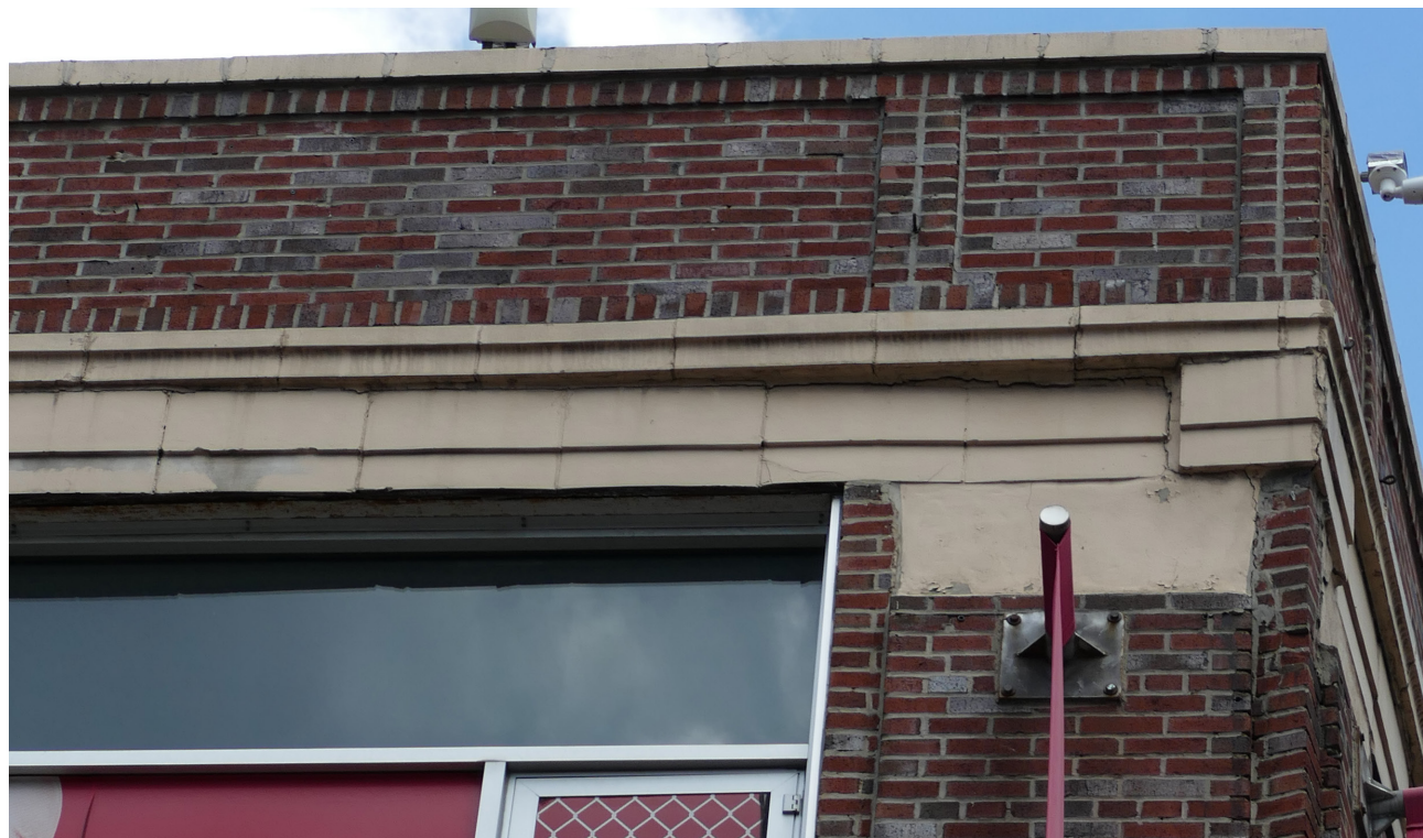
Missing terra-cotta capitals will be replicated and masonry displacement will be repaired.
