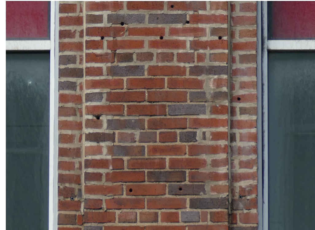
Holes in the existing brick will be repaired; incompatible pointing mortar will be removed and repointed to match historic.
