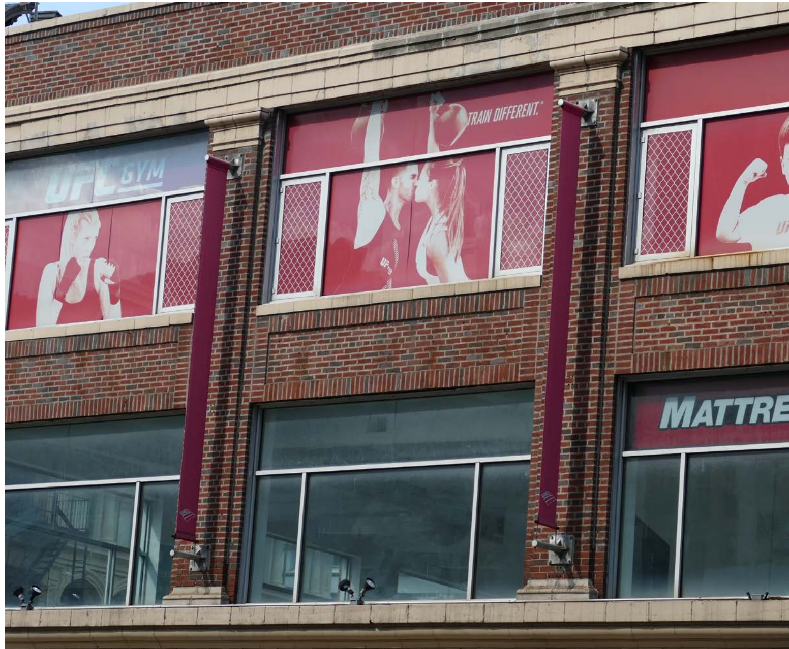
The existing windows are non-historic aluminum and do not match the historic configuration.
