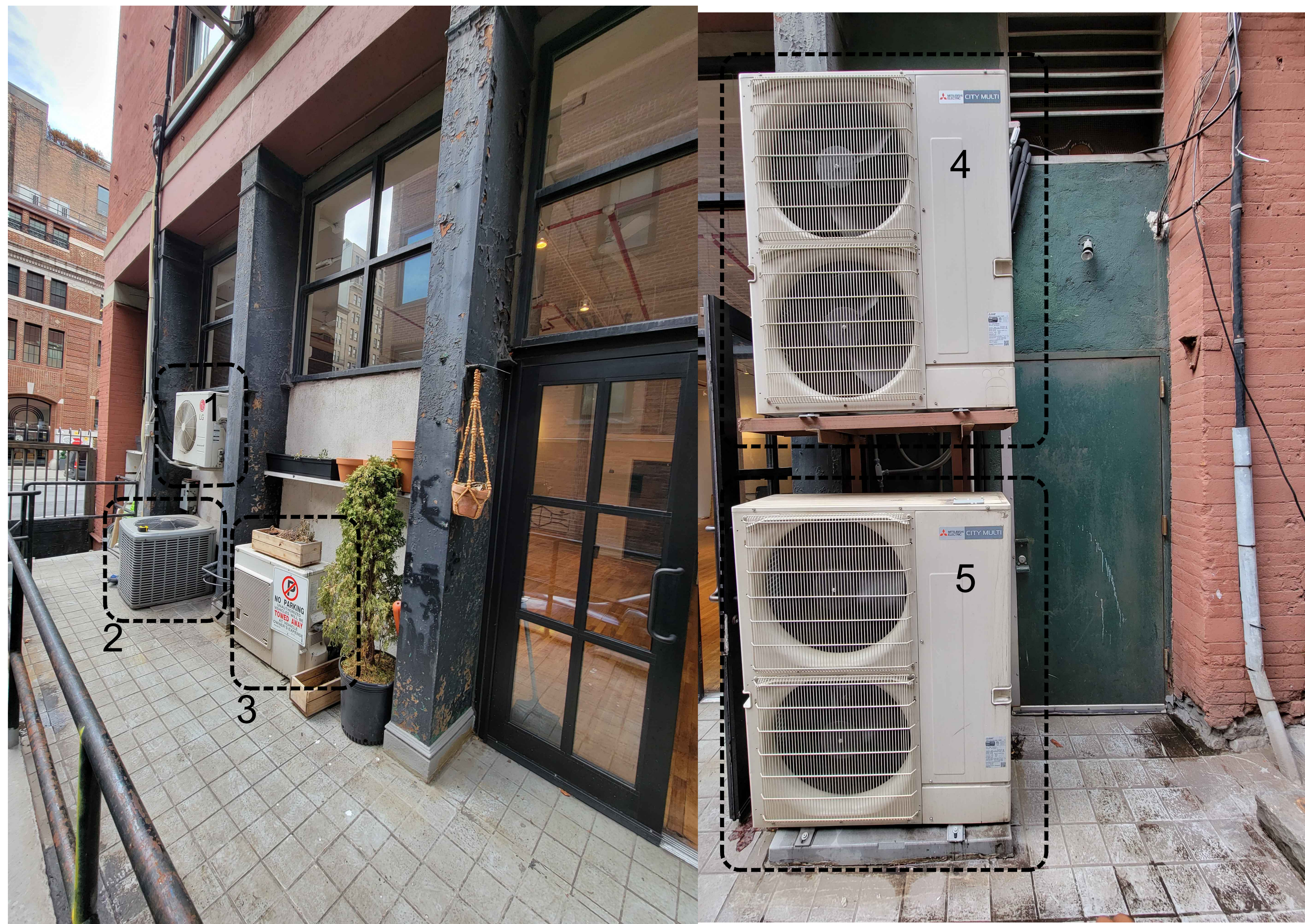
1 LOCATION #4 : VIOLATION - 160325 A-004 SCALE: N/A
