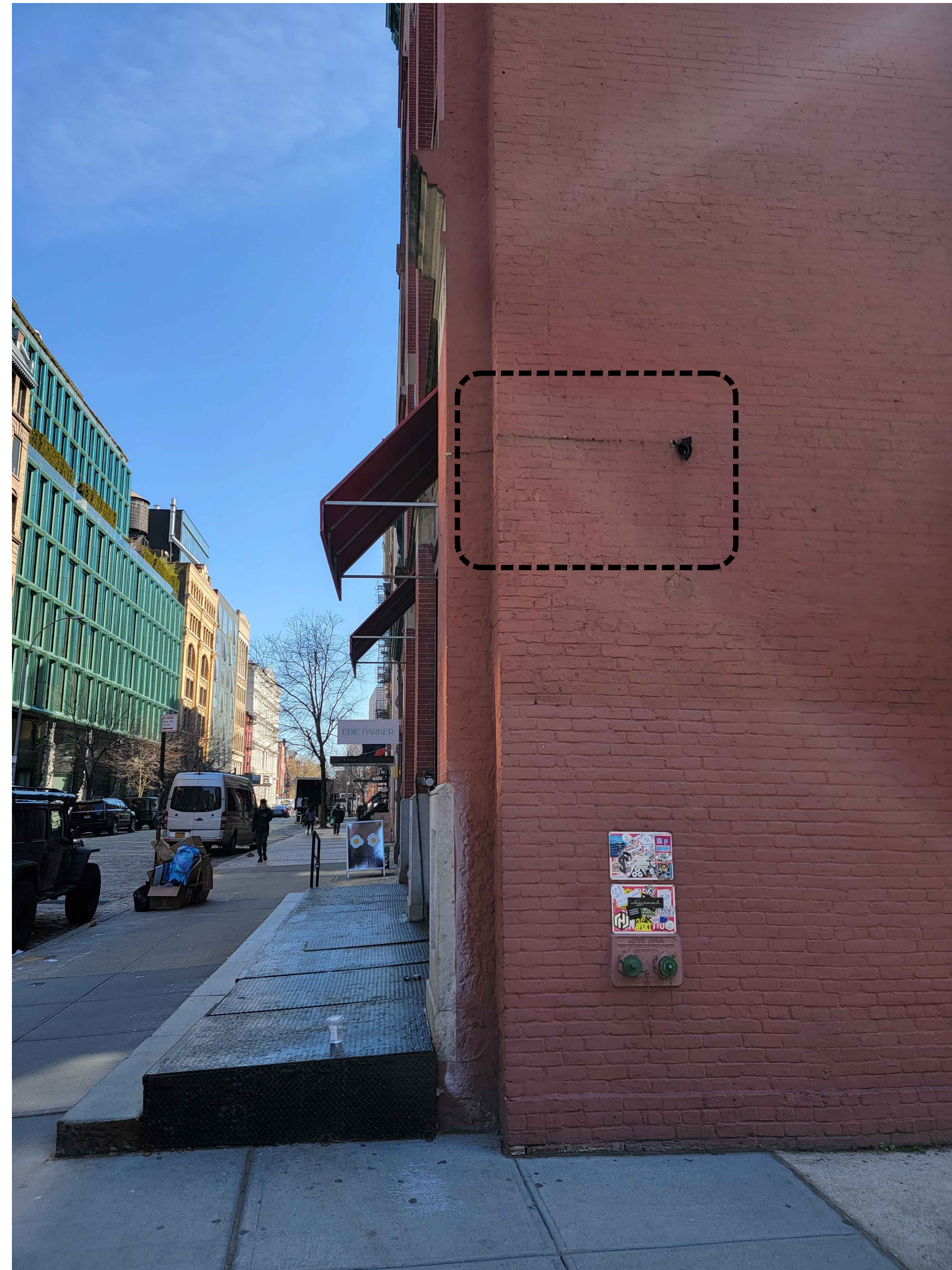
3 LOCATION #2 : VIOLATION - 160323 REMOVED A-005 SCALE: N/A
