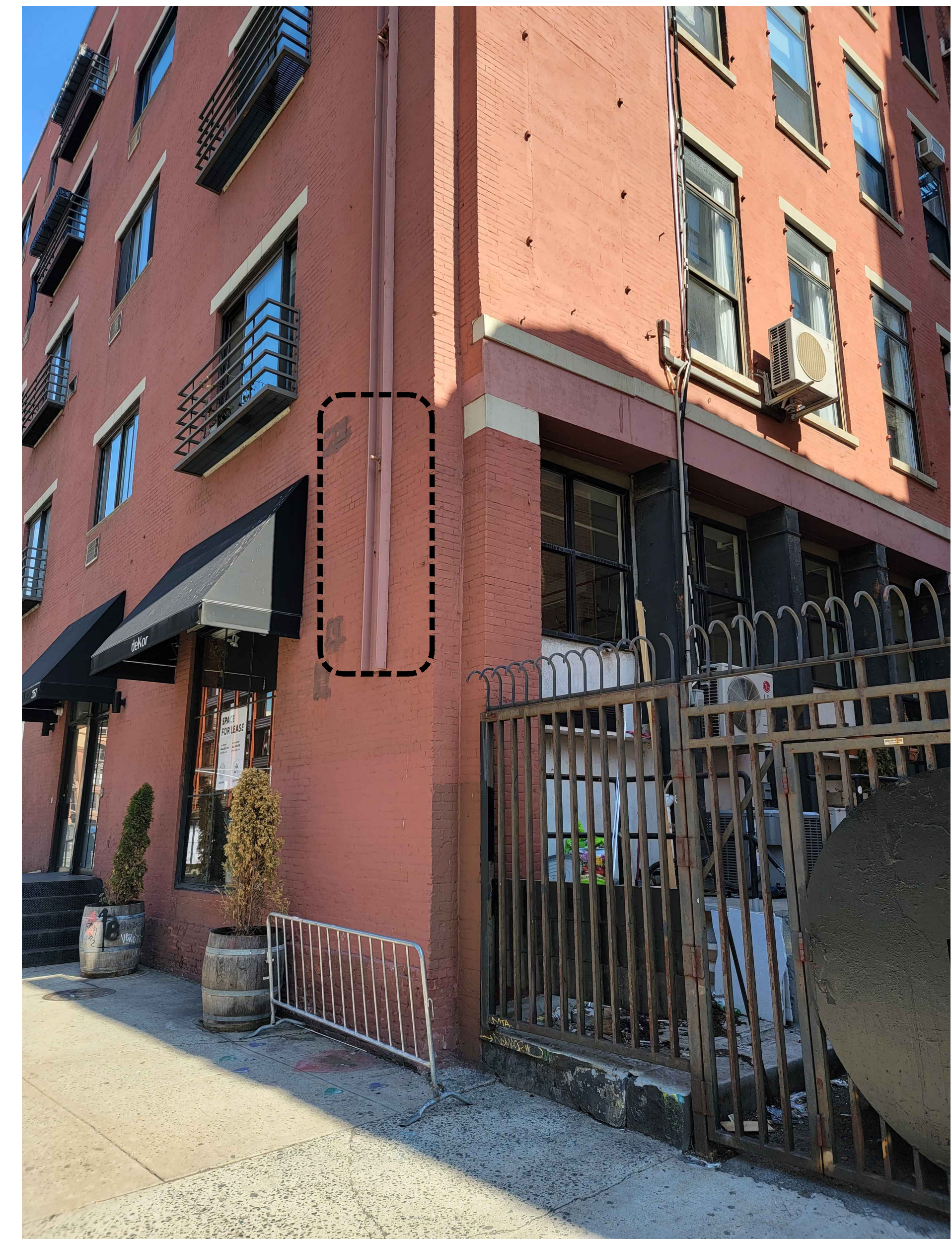
4 LOCATION #3 : VIOLATION - 160324 REMOVED A-005 SCALE: N/A
