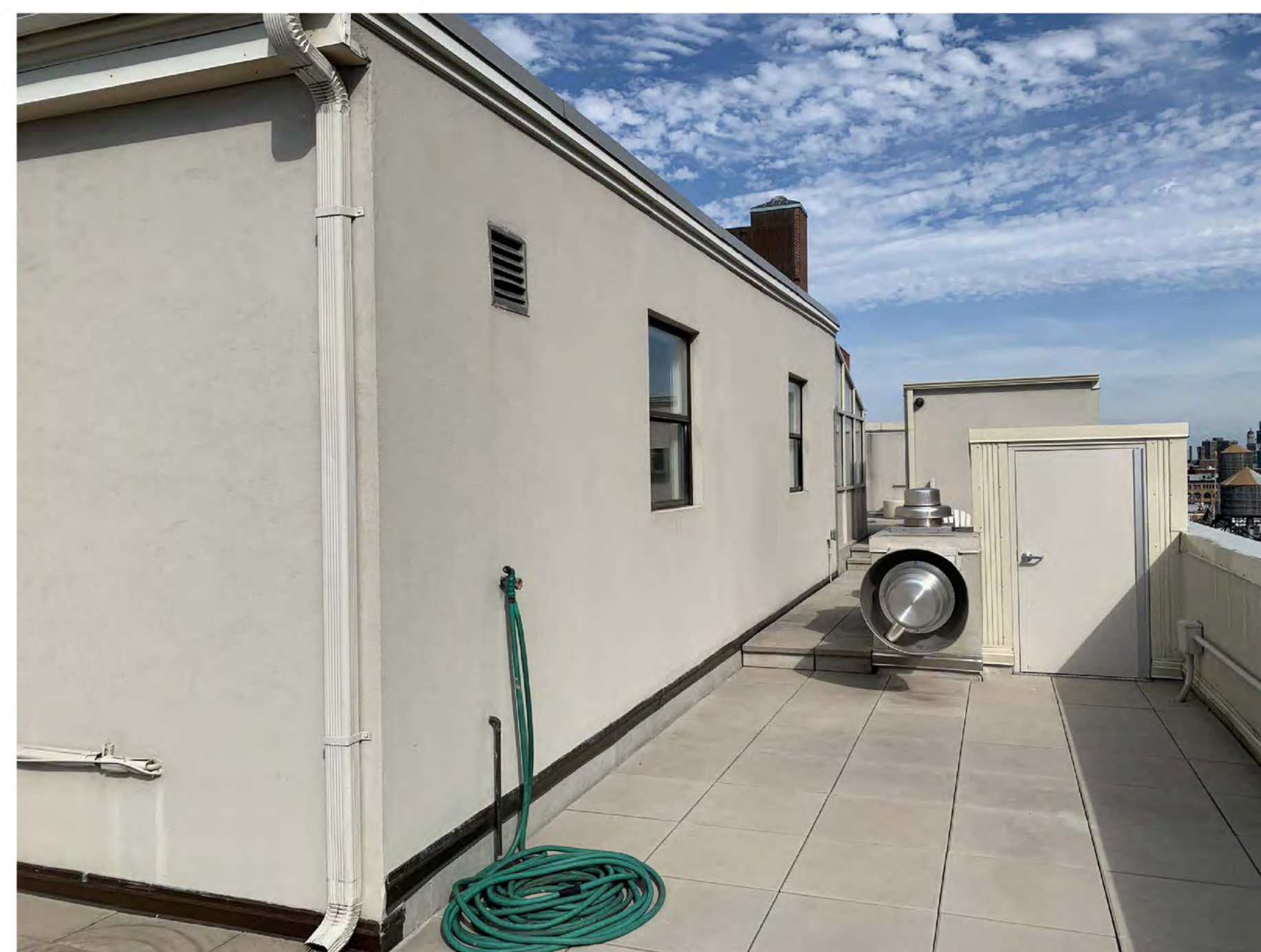
EXISTING EXHAUST VENTS & FANS
