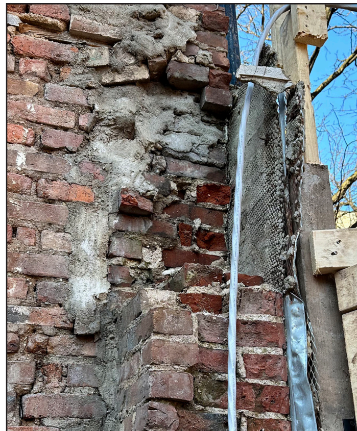
SIDE PROBE SHOWING REPLACED BRICK FACADE
