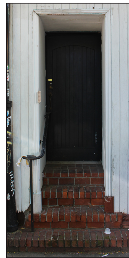
UNUSED SECONDARY ENTRY DOOR
