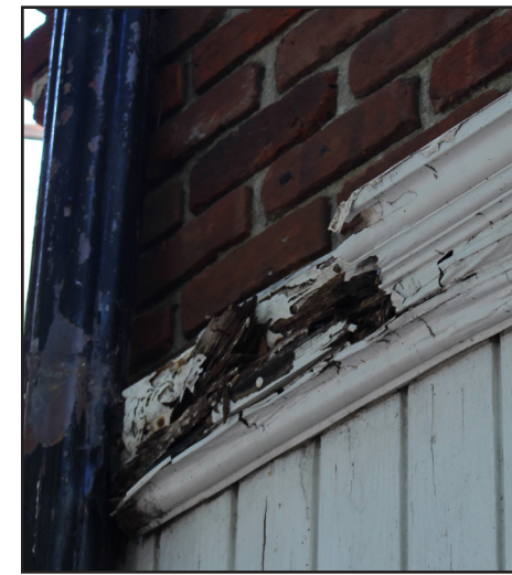
DETERIORATED FIRST FLOOR WOOD PANELING
