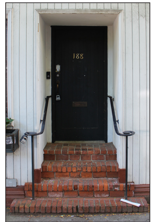
PRIMARY ENTRY DOOR
