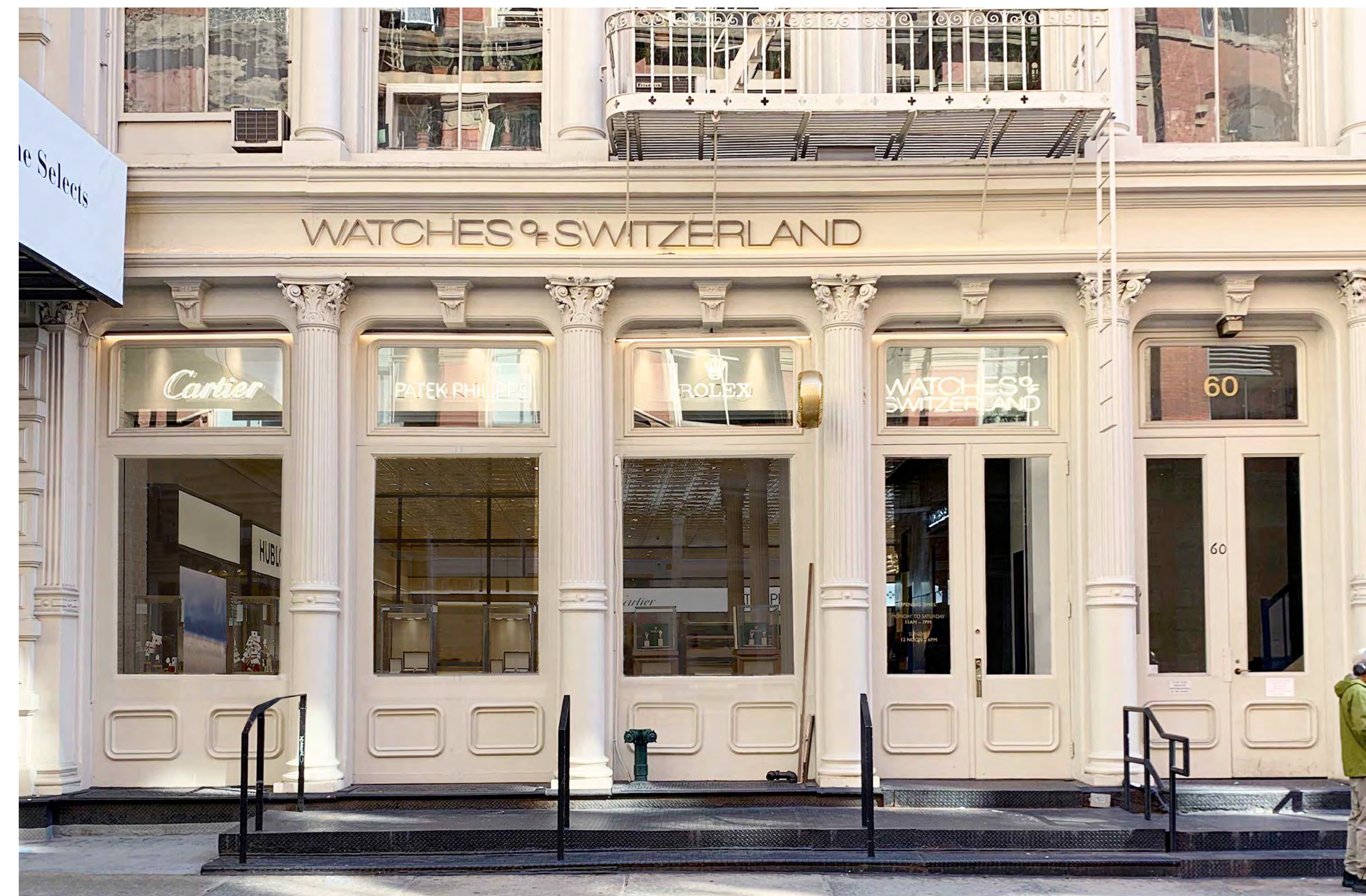
BAY 01 ORIGINAL CAST IRON BASE BAY 02 NEW BASE TO MATCH EXISTING CAST IRON BASE BAY 03 ORIGINAL CAST IRON BASE BAY 04 NEW DOORS TO MATCH EXISTING BAY 05 EXISTING WOOD DOORS
