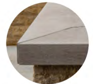
PRECAST CONCRETE COPING
