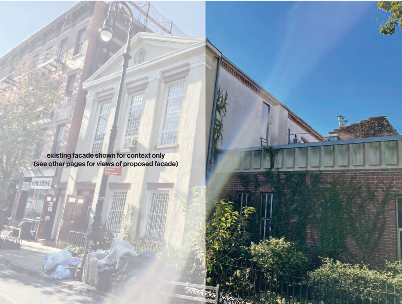
STREET VIEW SHOWING ROOFTOP MECHANICAL EQUIPMENT & SIDE WALL OPENINGS
