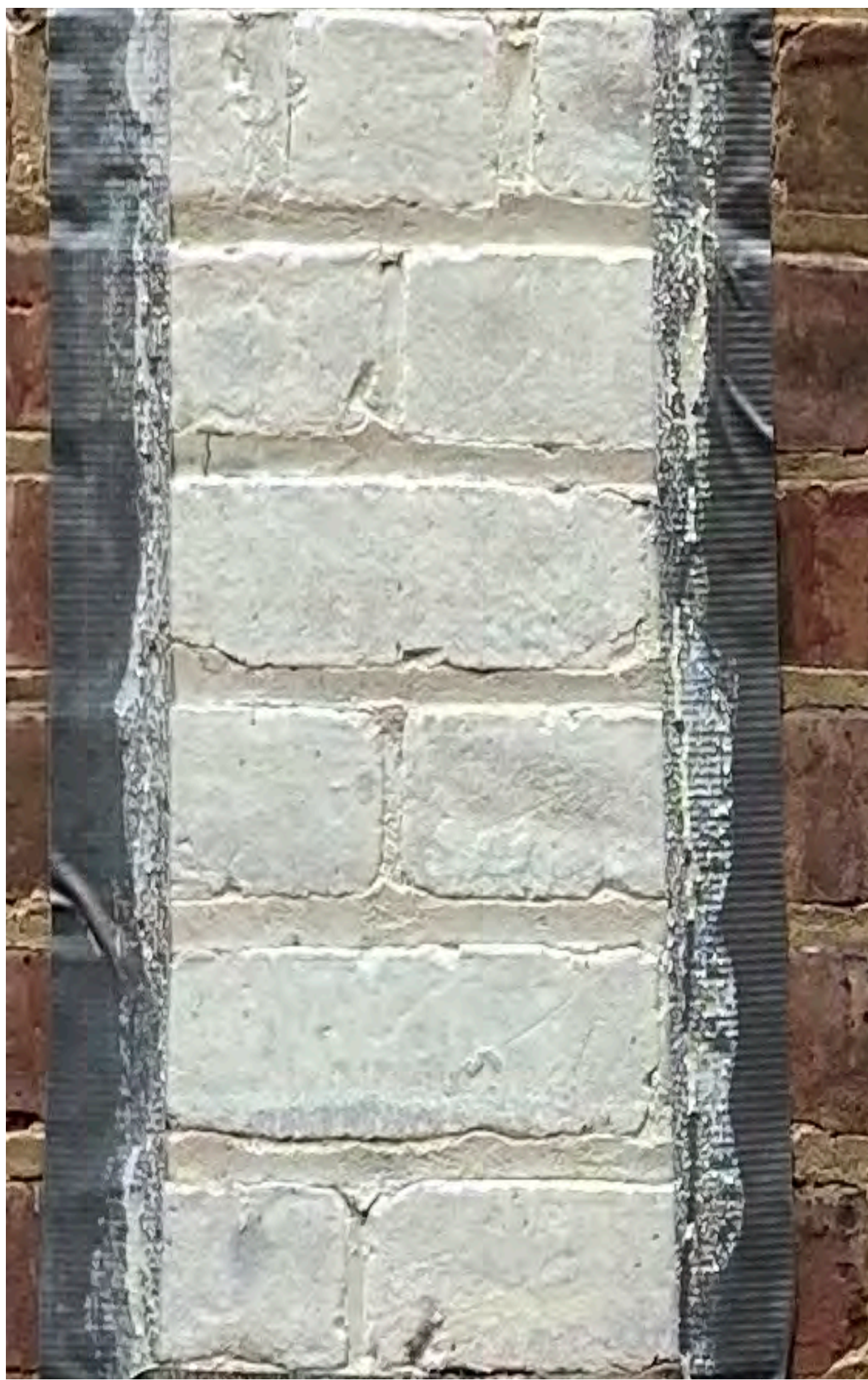
BRICK STAIN TESTS AT EXISTING COURTYARD WALL (KEIM COLOR NO. 9078 / 1:5 DILUTION RATIO)
