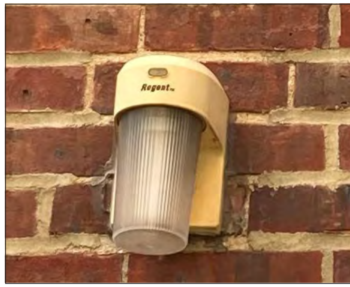
EXISTING LIGHT AT BUILDING ENTRY (NOT AN ORIGINAL) TO BE REPLACED.
