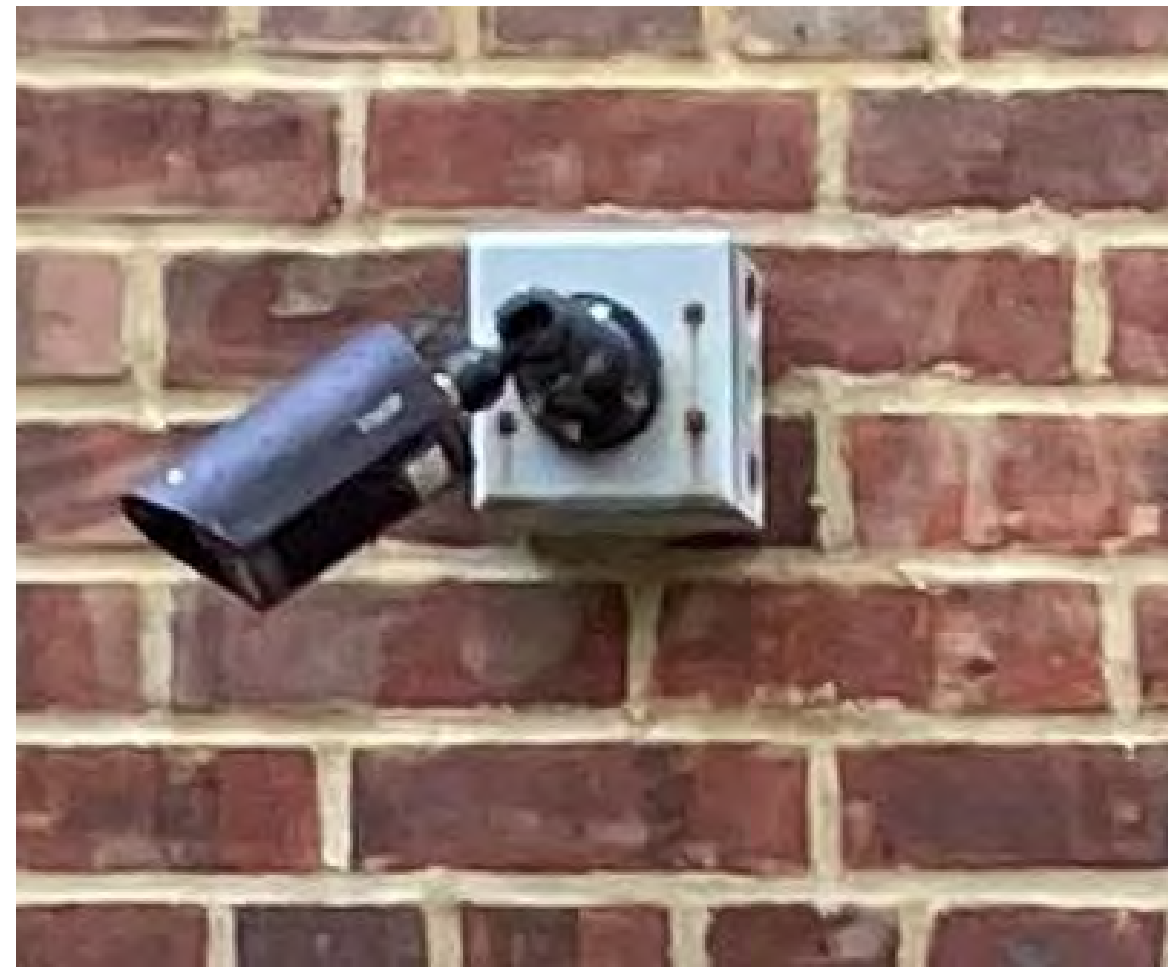
EXISTING SECURITY CAMERA TO BE REPLACED
