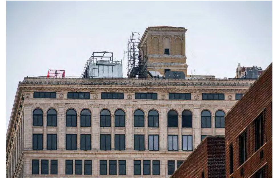
③ GENERATOR MOCK-UP PHOTO - ENLARGED NTS
