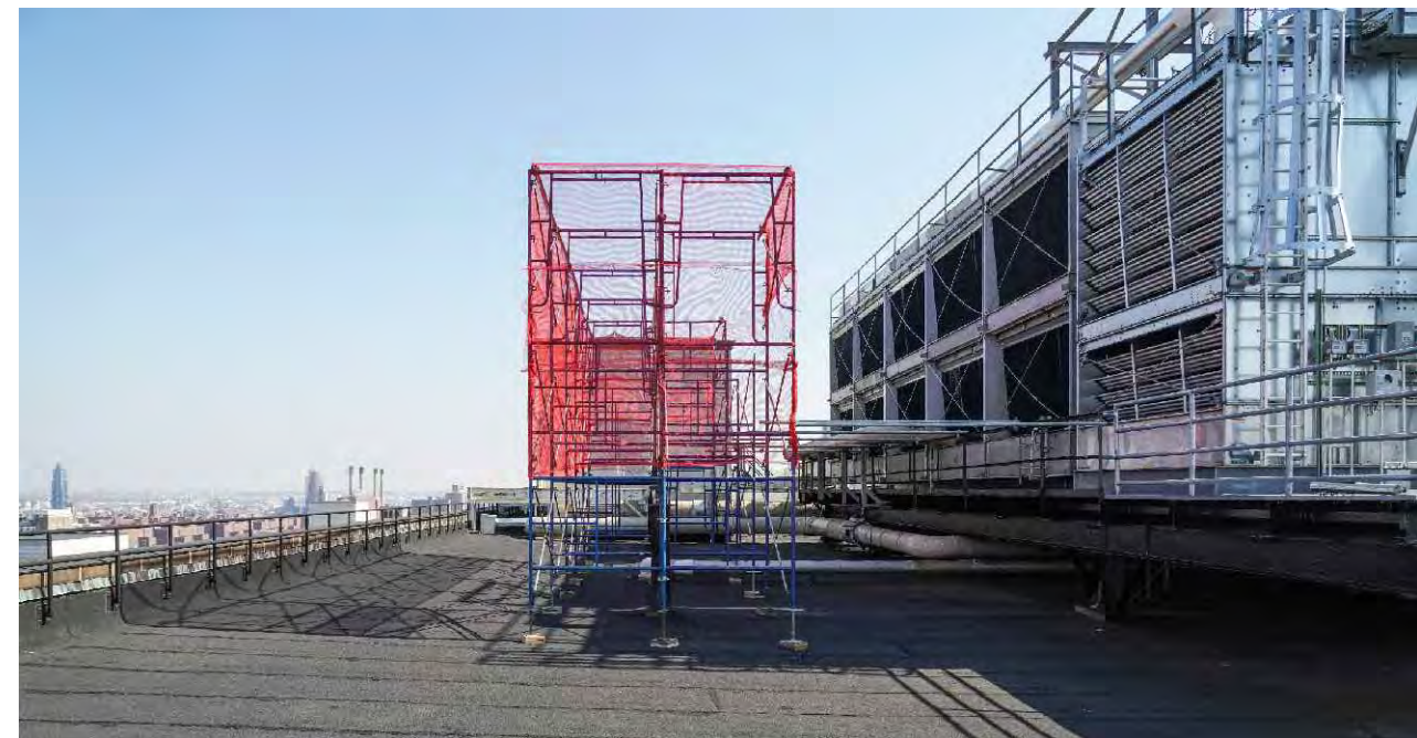
2 GENERATOR MOCK-UP PHOTO FROM ROOF NTS
