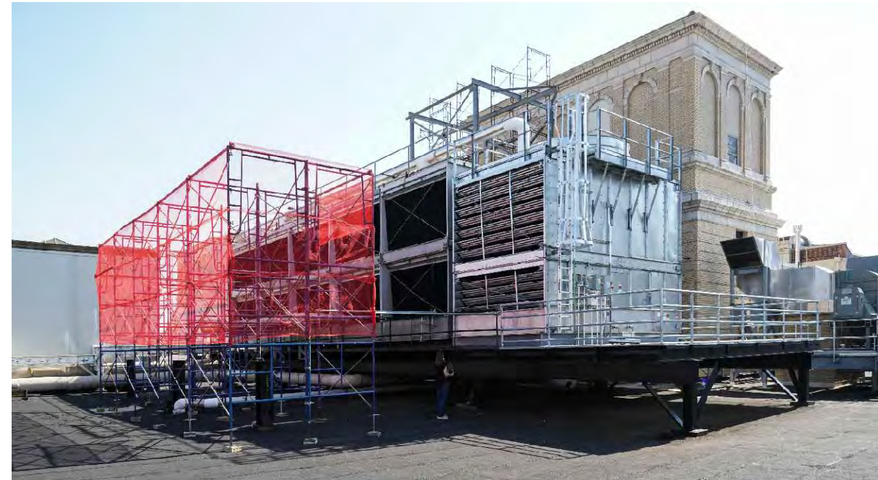
1 GENERATOR MOCK-UP PHOTO FROM ROOF NTS
