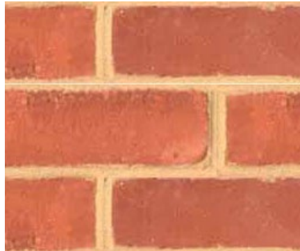
EXISTING REAR FACADE WALL: STILES AND HART BRICK COMPANY LIGHT RED WATERSTRUCK
