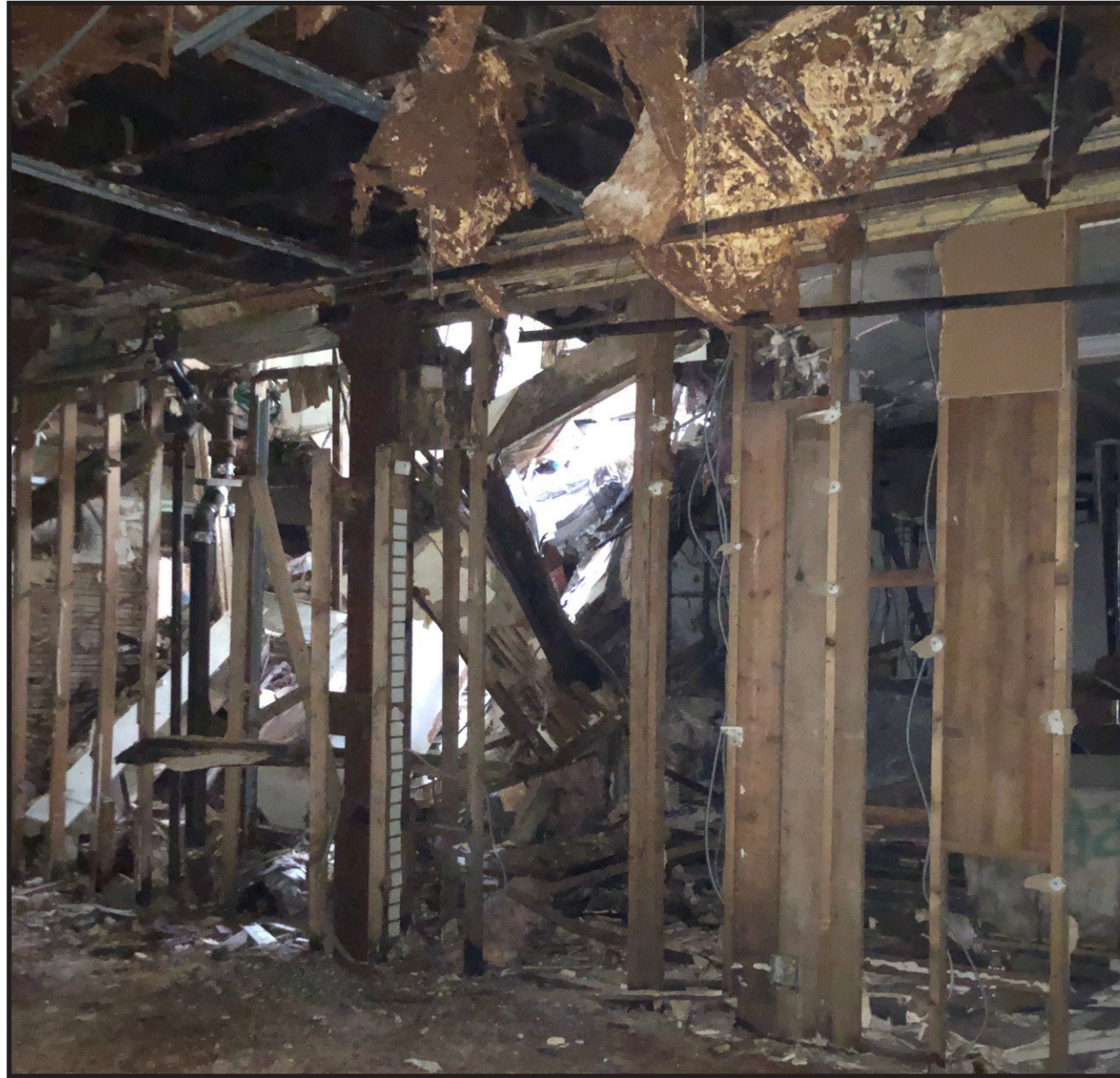
PARTIAL ROOF COLLAPSE (JUNE 17, 2020)
