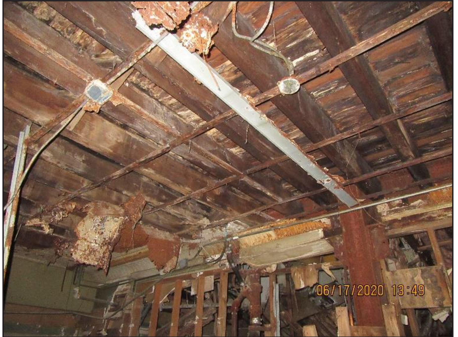
CORRODED STEEL COLUMNS AND GIRDER @ FIRST FLOOR (JUNE 17, 2020)
