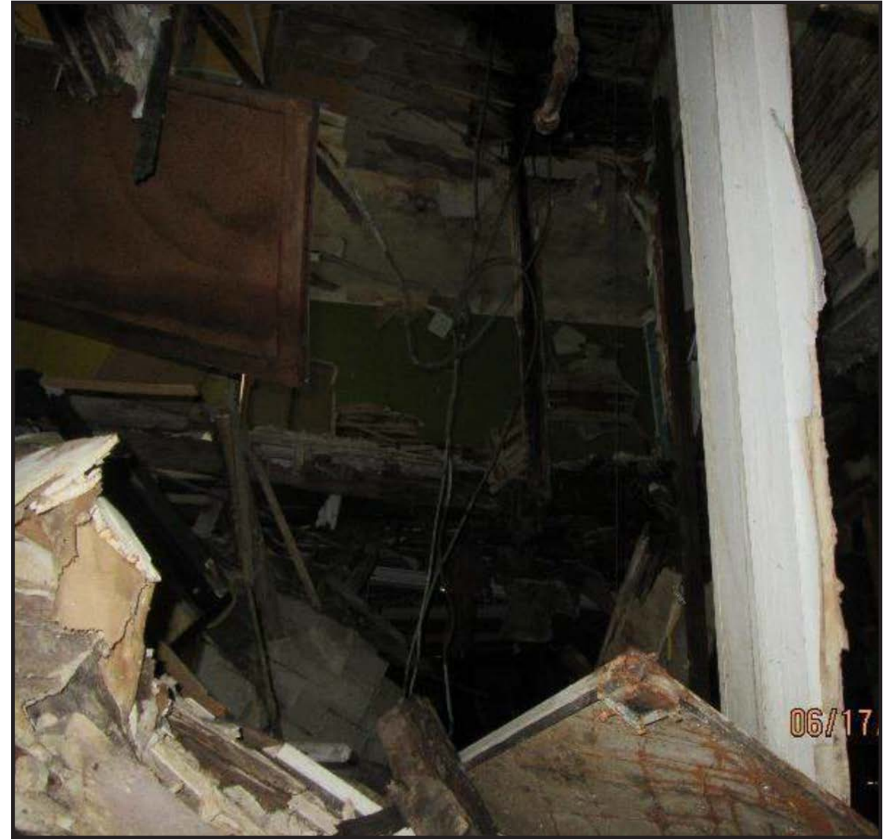
PARTIAL 2ND FLOOR COLLAPSE (JUNE 17, 2020)
