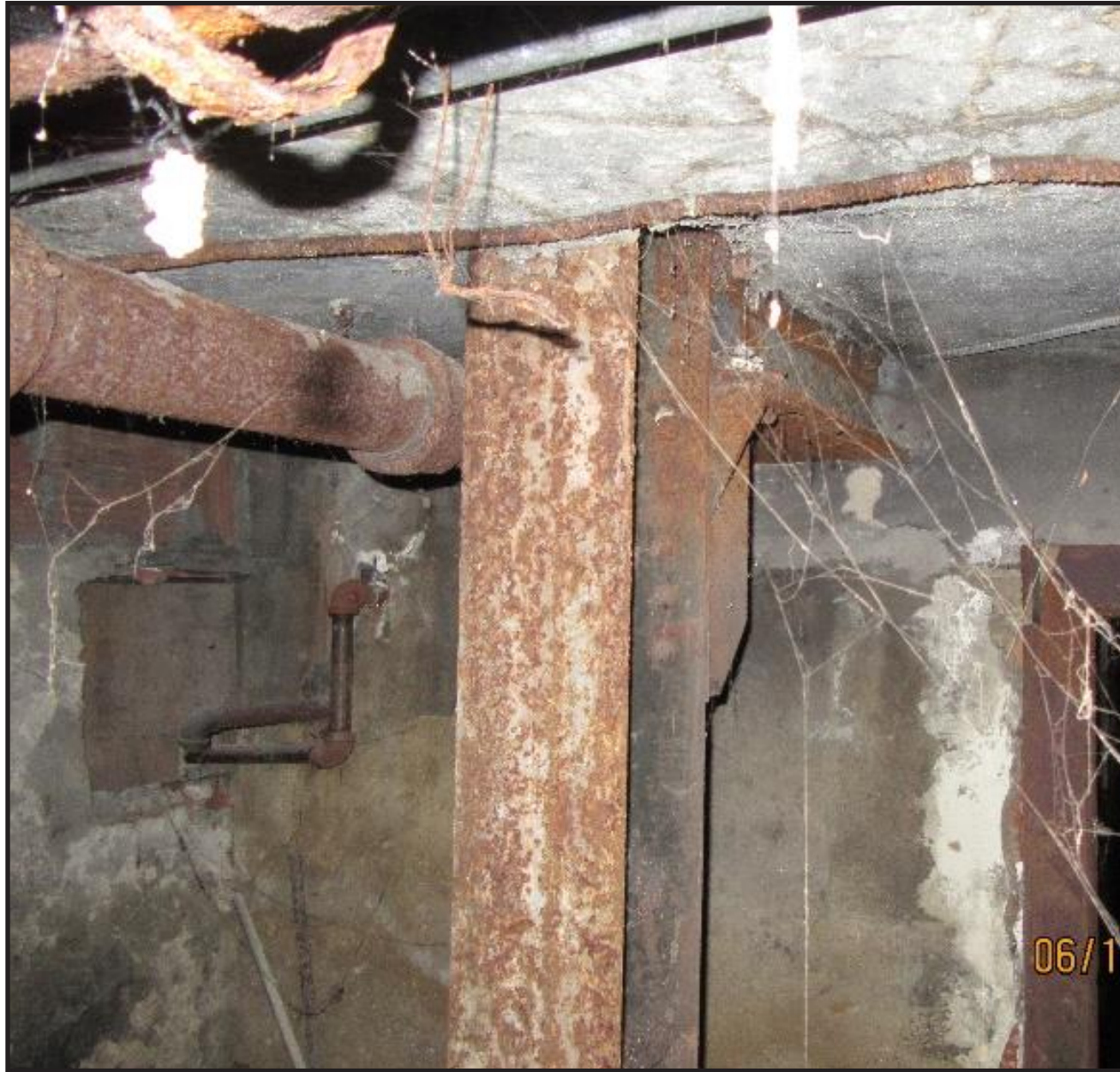
CORRODED STEEL STRUCTURE AT CELLAR (JUNE 17, 2020)
