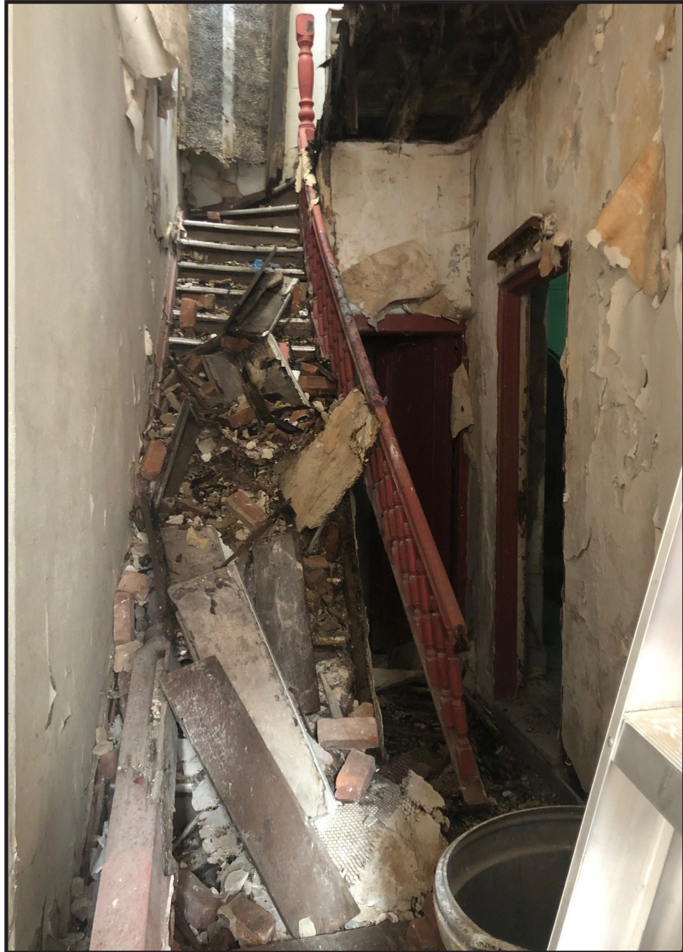
PARTIALLY COLLAPSED FIRST FLOOR STAIR (JUNE 17, 2020)
