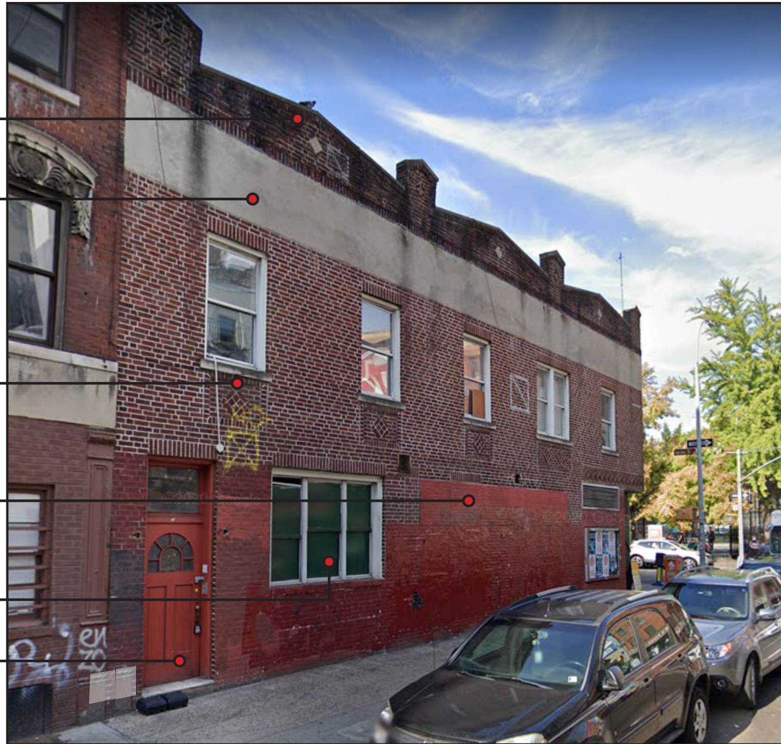
CURRENT: EAST FACADE
