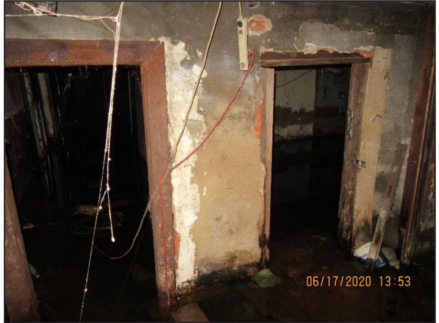
PARTIALLY FLOODED CELLAR (JUNE 17, 2020)
