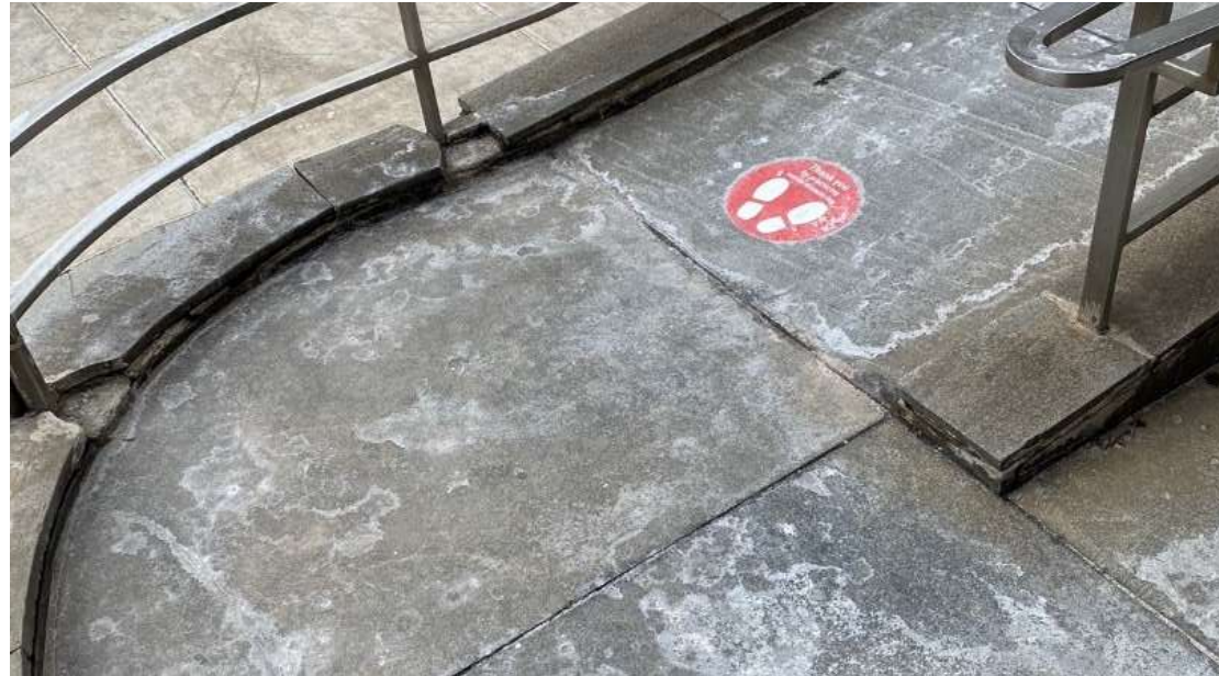
1 – Existing ramp damage
