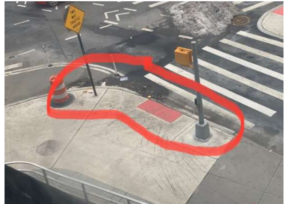
3 – Ponding in crosswalk – to be addressed by DOT
