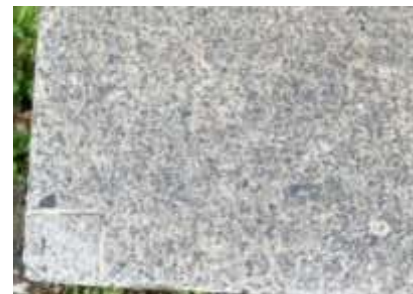
Stair treads and cheek walls – granite to match building base and existing stair on 7 th Ave.
