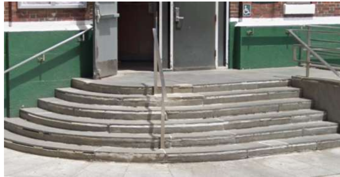
2 – Existing stair damage
