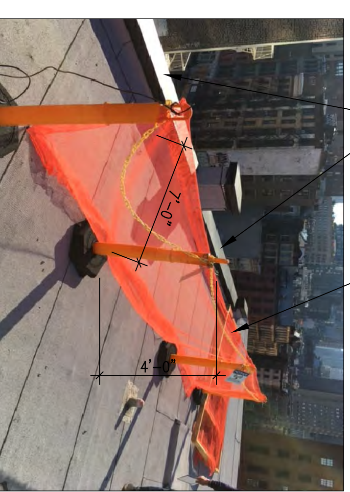
EXISTING LOW PARAPET TO REMAIN PROPOSED MOCK UP OF PARAPET FENCE LOOKING SOUTH
