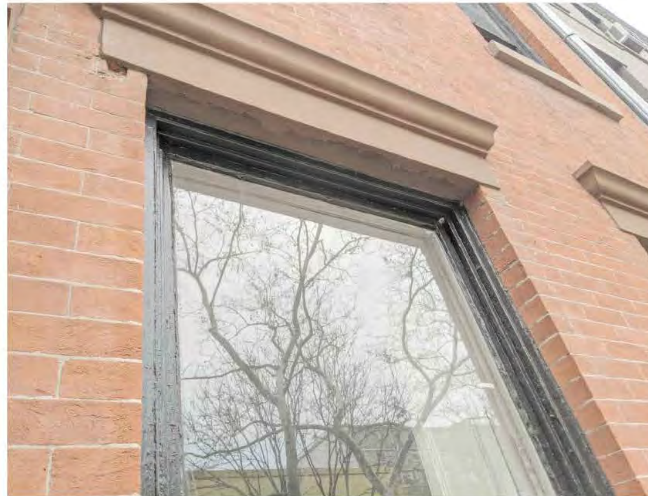
PHOTO OF FRONT FIRST FLOOR WINDOW (DATE OF PHOTO 03/03/20) NOT TO SCALE
