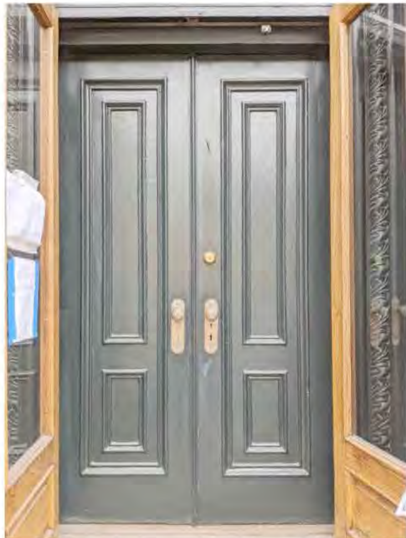
PHOTO OF EXISTING INNER ENTRY DOORS (DATE OF PHOTO 03/03/20) NOT TO SCALE
