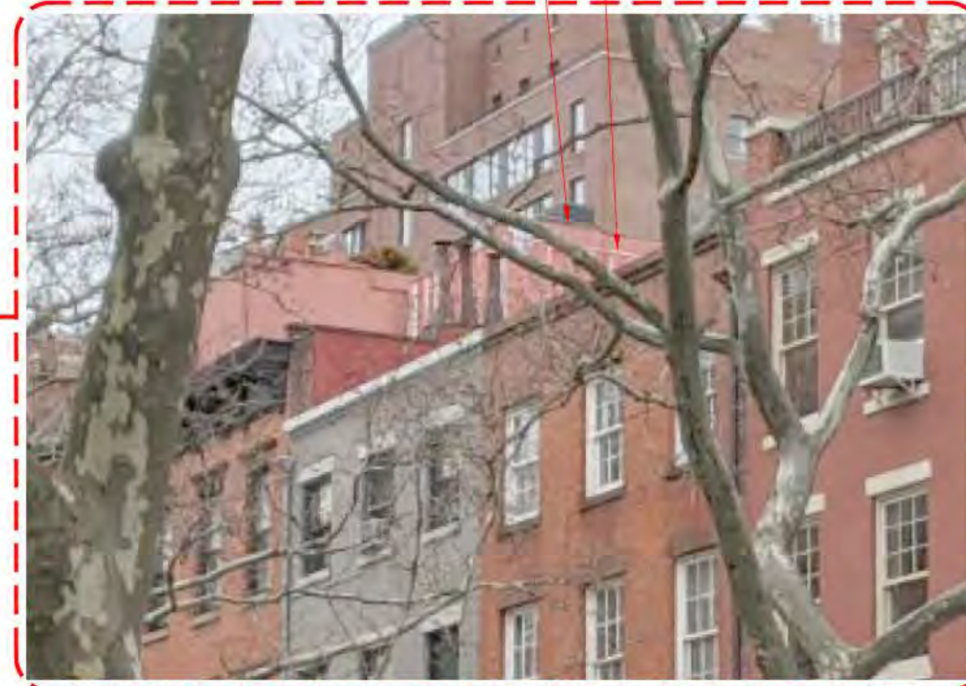
CLOSEUP PHOTO OF ROOF MOCKUP FROM STREET (DATE OF PHOTO 03/03/20) NOT TO SCALE
