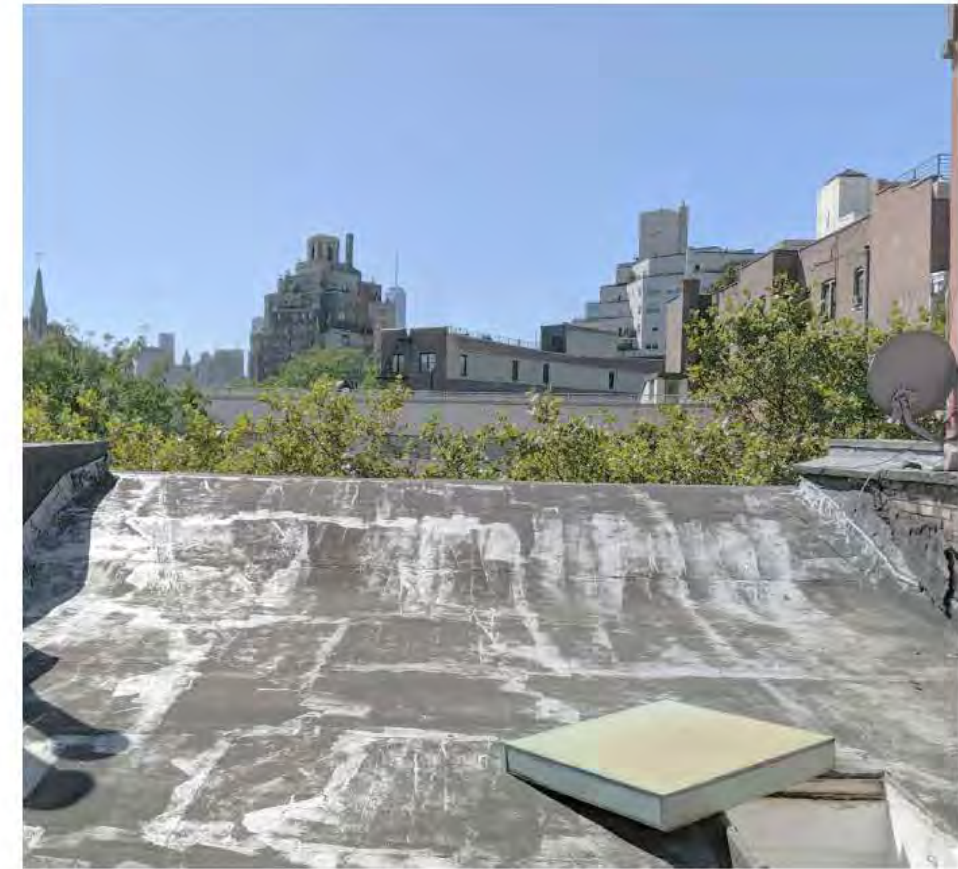
PHOTO OF ROOF - LOOKING SOUTH 'B' (DATE OF PHOTO 09/17/19) NOT TO SCALE
