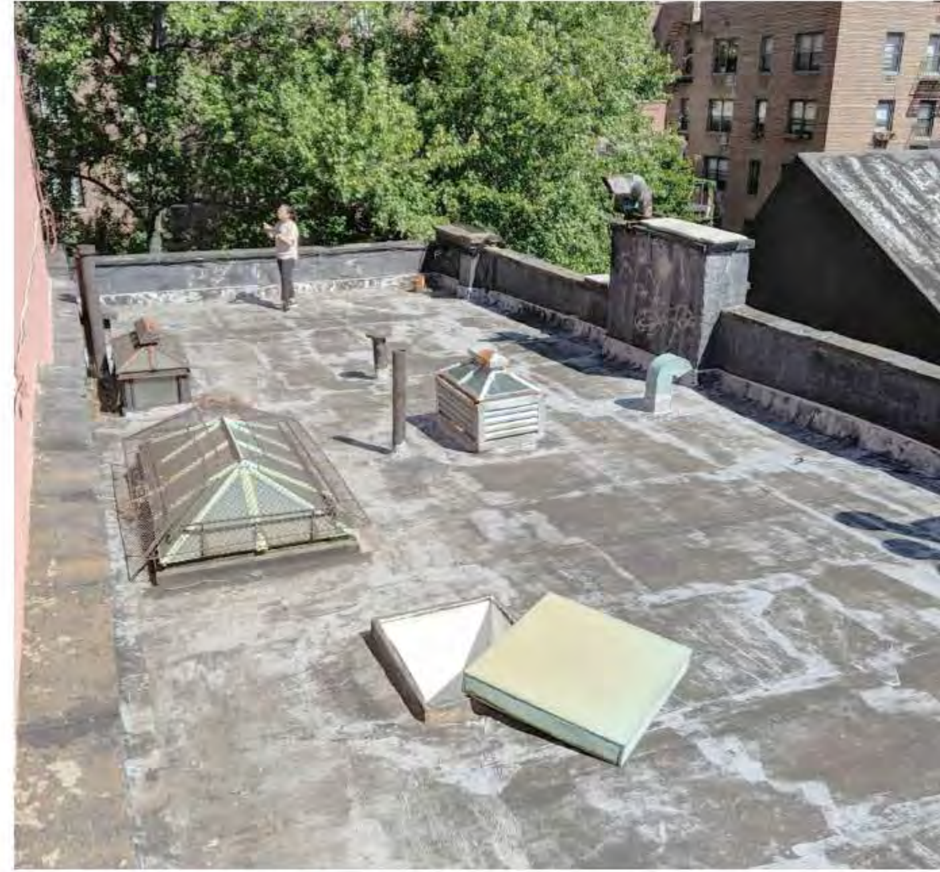
PHOTO OF SKYLIGHTS, FLUES, AND ROOF HATCH (DATE OF PHOTO 09/17/19) NOT TO SCALE
