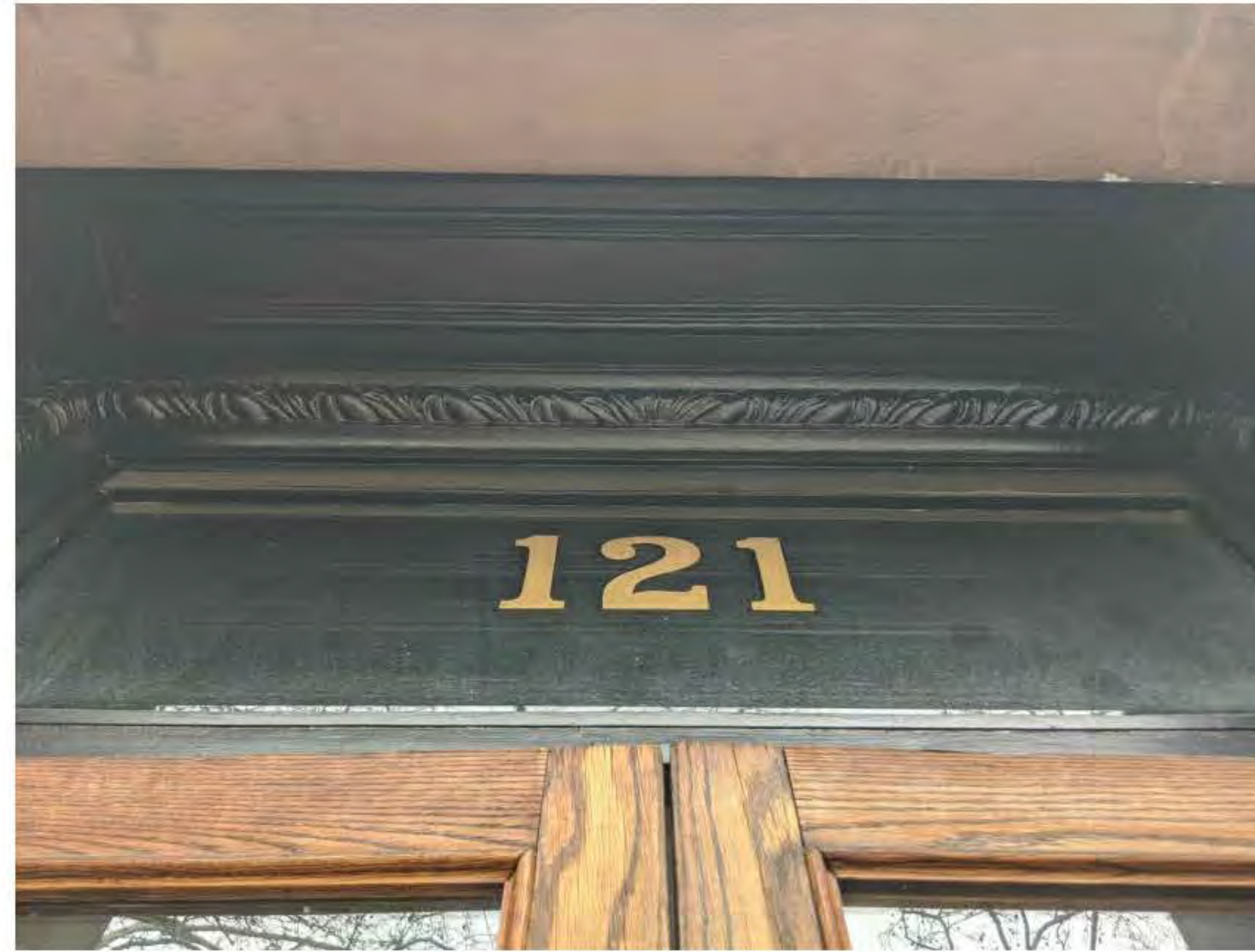
CLOSE UP OF EXISTING SOFFIT OVER ENTRY DOORS (DATE OF PHOTO 03/03/20) NOT TO SCALE
