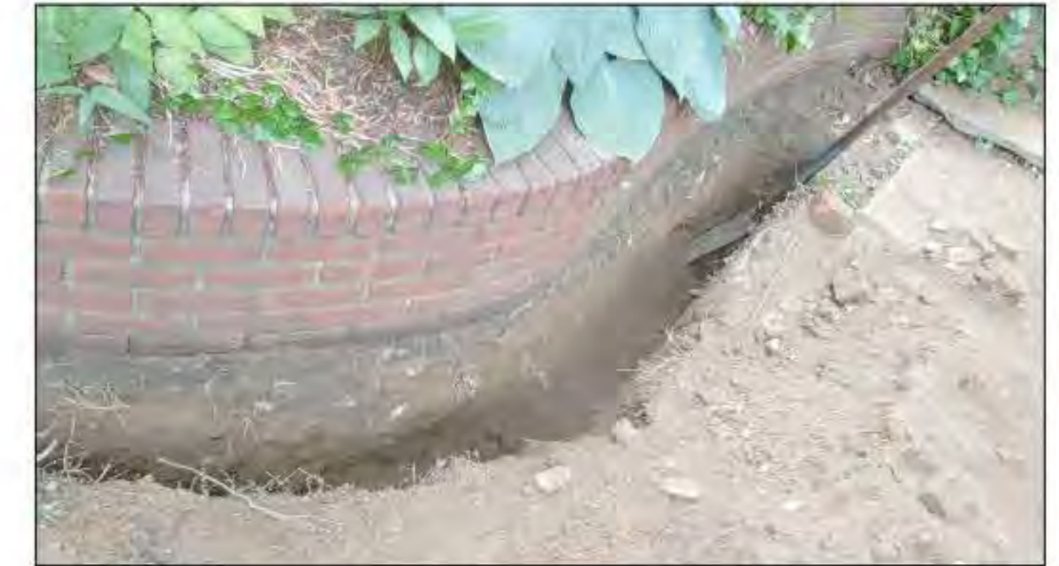
PHOTO OF TREE ROOT EXCAVATION 'A' (DATE OF PHOTO 06/30/20) NOT TO SCALE
