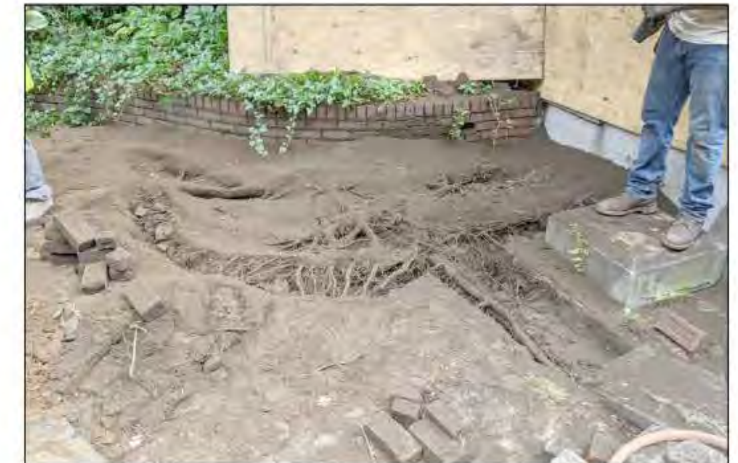
PHOTO OF TREE ROOT EXCAVATION 'B' (DATE OF PHOTO 06/30/20) NOT TO SCALE
