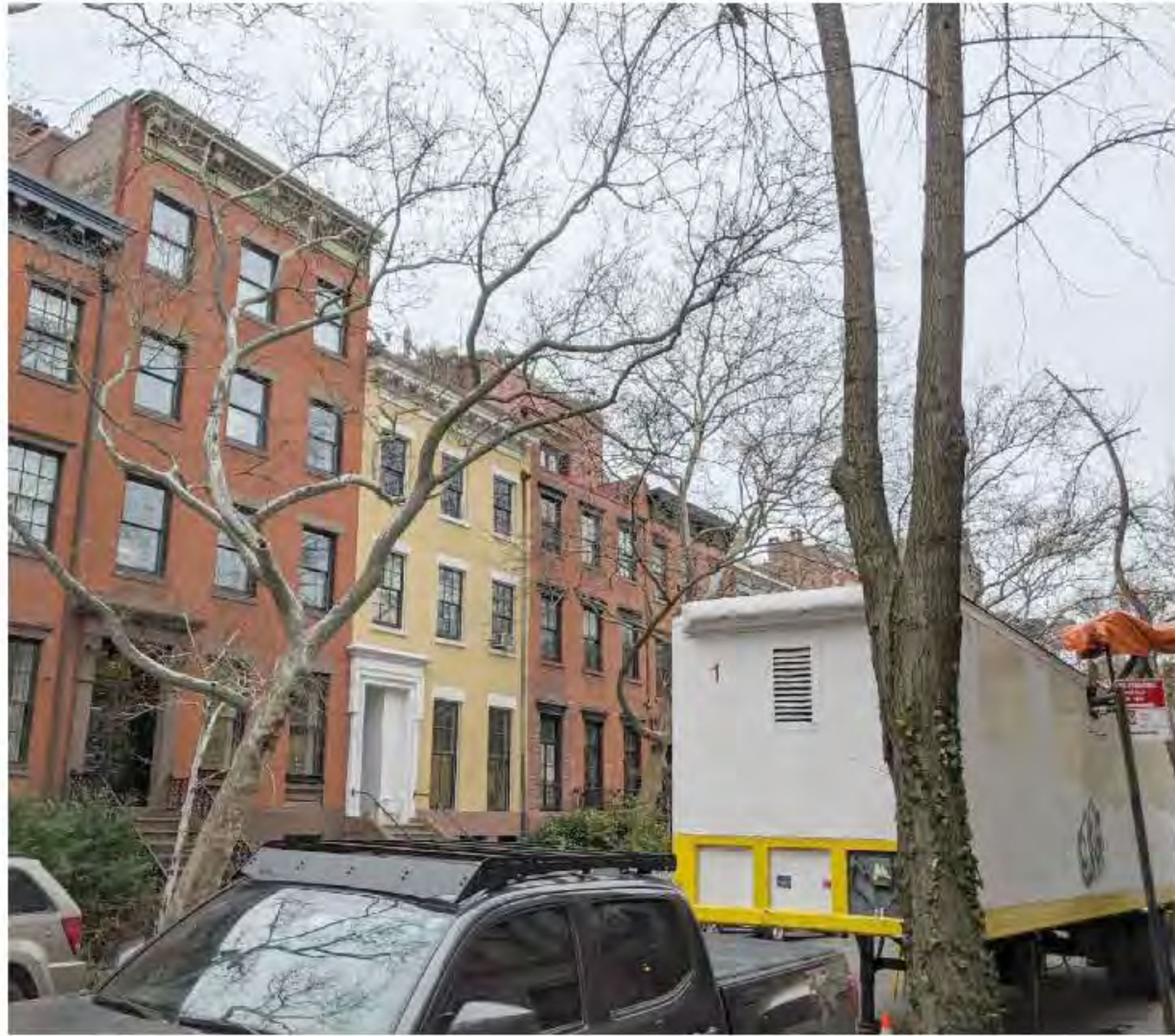
PHOTO OF ROOF MOCKUP FROM STREET 'A' (DATE OF PHOTO 03/03/20) NOT TO SCALE
