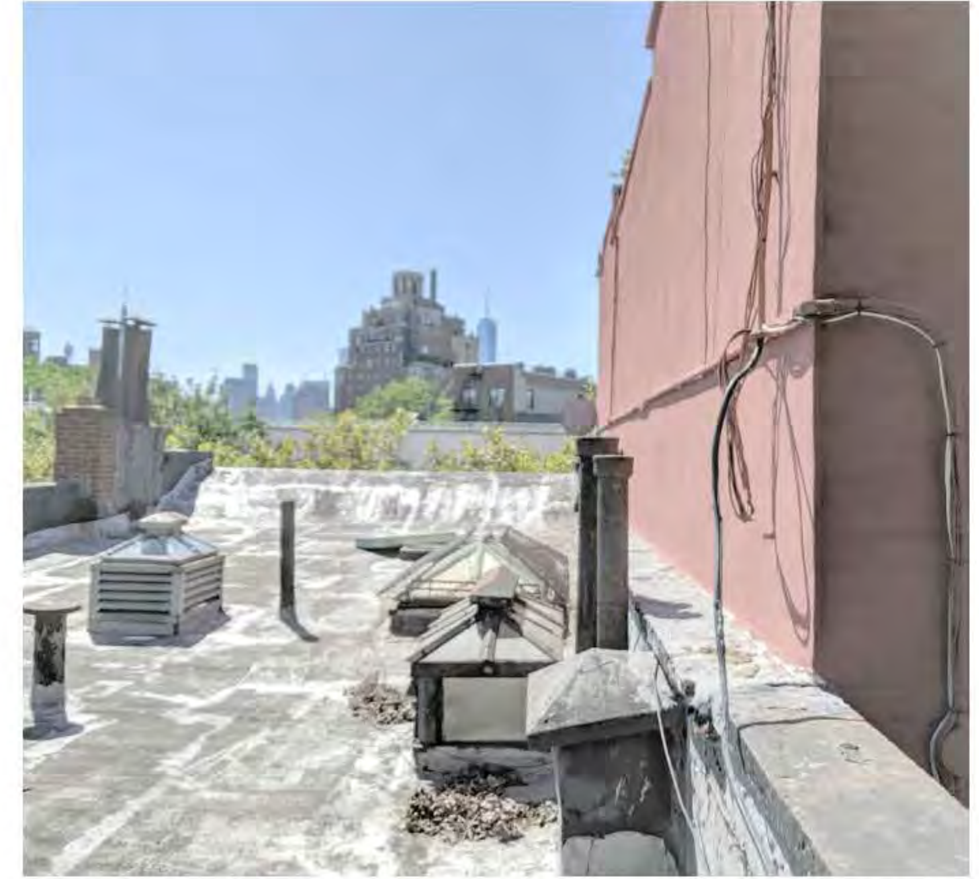
PHOTO OF SKYLIGHTS, FLUES, HATCH AND WEST PARAPET (DATE OF PHOTO 09/17/19) NOT TO SCALE
