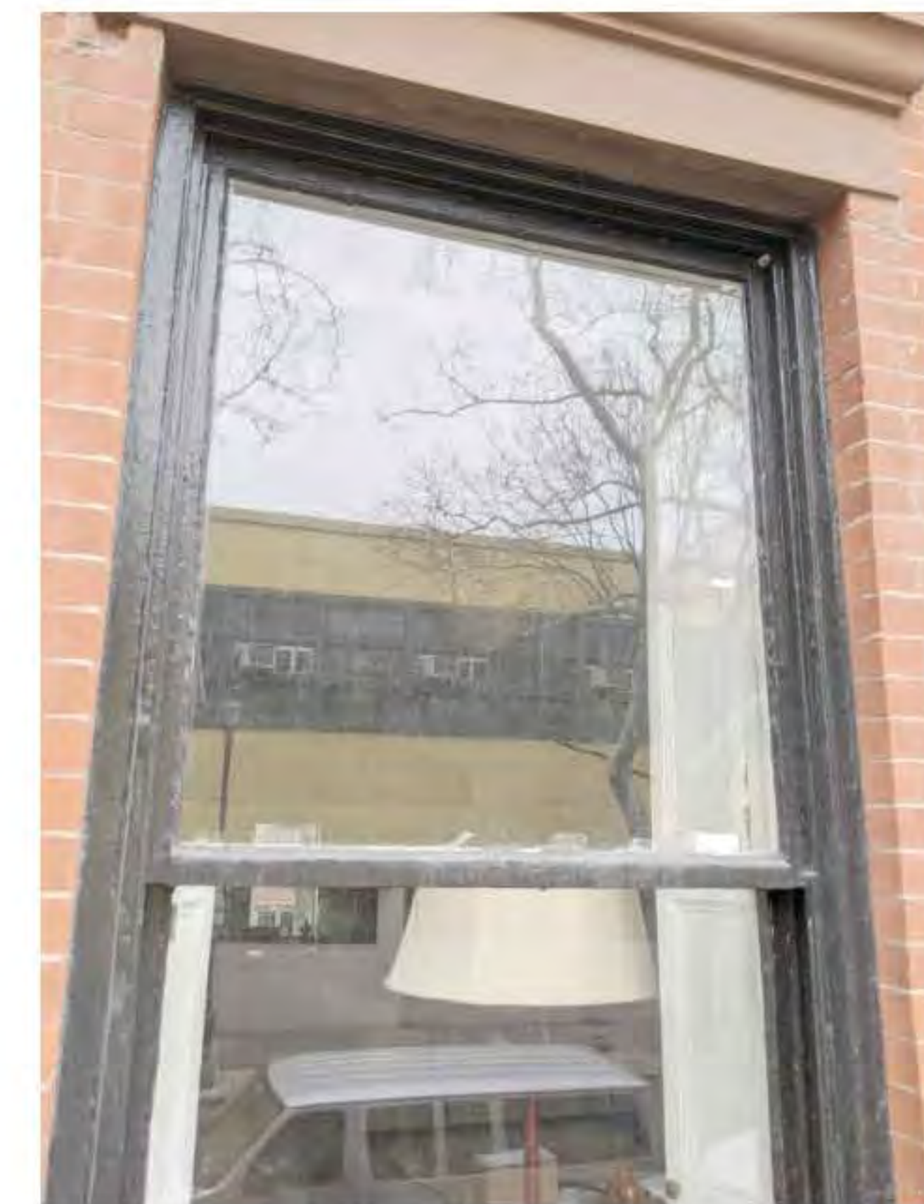
PHOTO OF FRONT FIRST FLOOR WINDOW (DATE OF PHOTO 03/03/20) NOT TO SCALE
