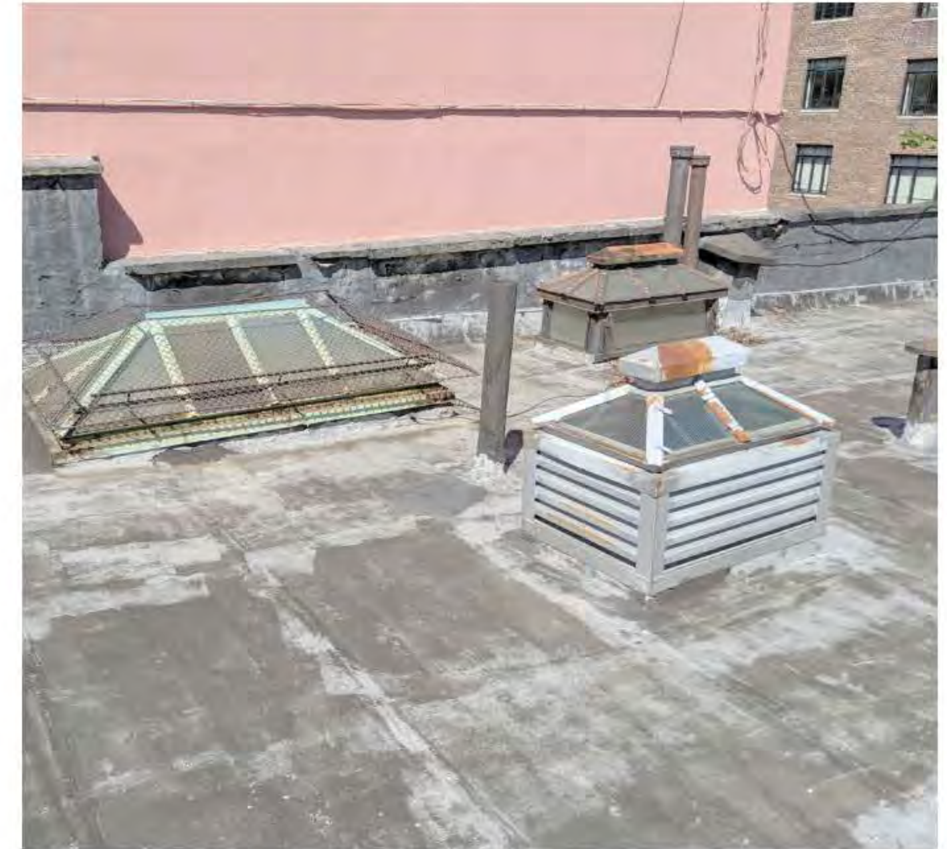
PHOTO OF SKYLIGHTS, FLUES, AND ROOF HATCH (DATE OF PHOTO 09/17/19) NOT TO SCALE
