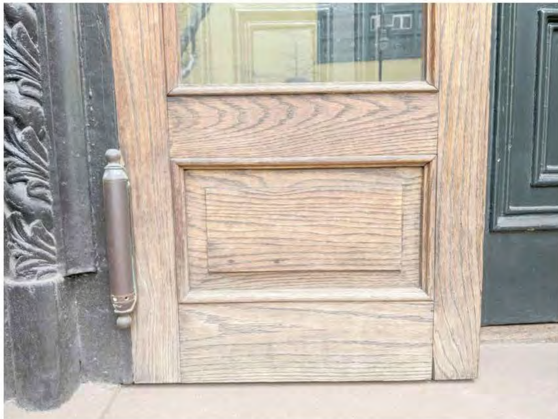
CLOSE UP OF EXISTING ENTRY DOOR HINGE (DATE OF PHOTO 03/03/20) NOT TO SCALE
