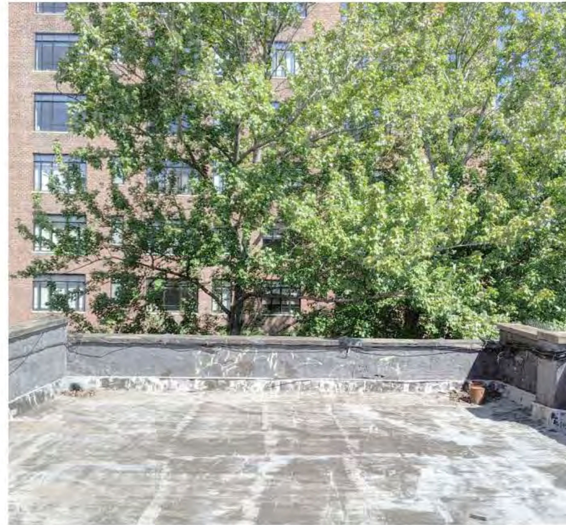
PHOTO OF ROOF - LOOKING NORTH 'A' (DATE OF PHOTO 09/17/19) NOT TO SCALE
