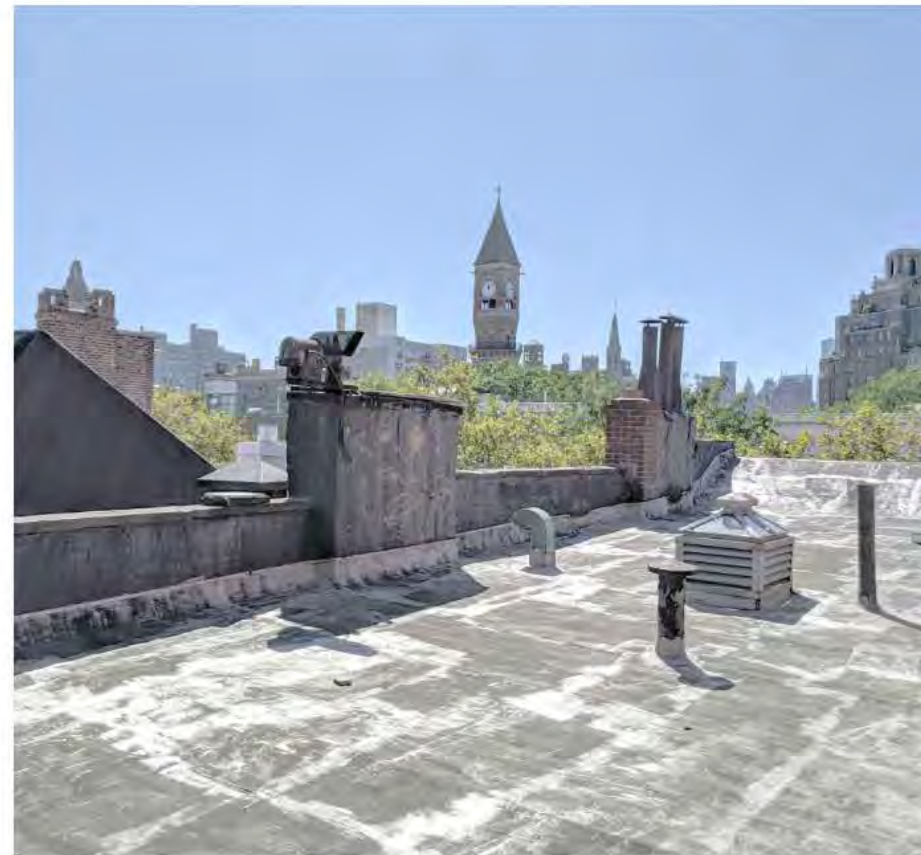
PHOTO OF ROOF - LOOKING EAST 'C' (DATE OF PHOTO 09/17/19) NOT TO SCALE
