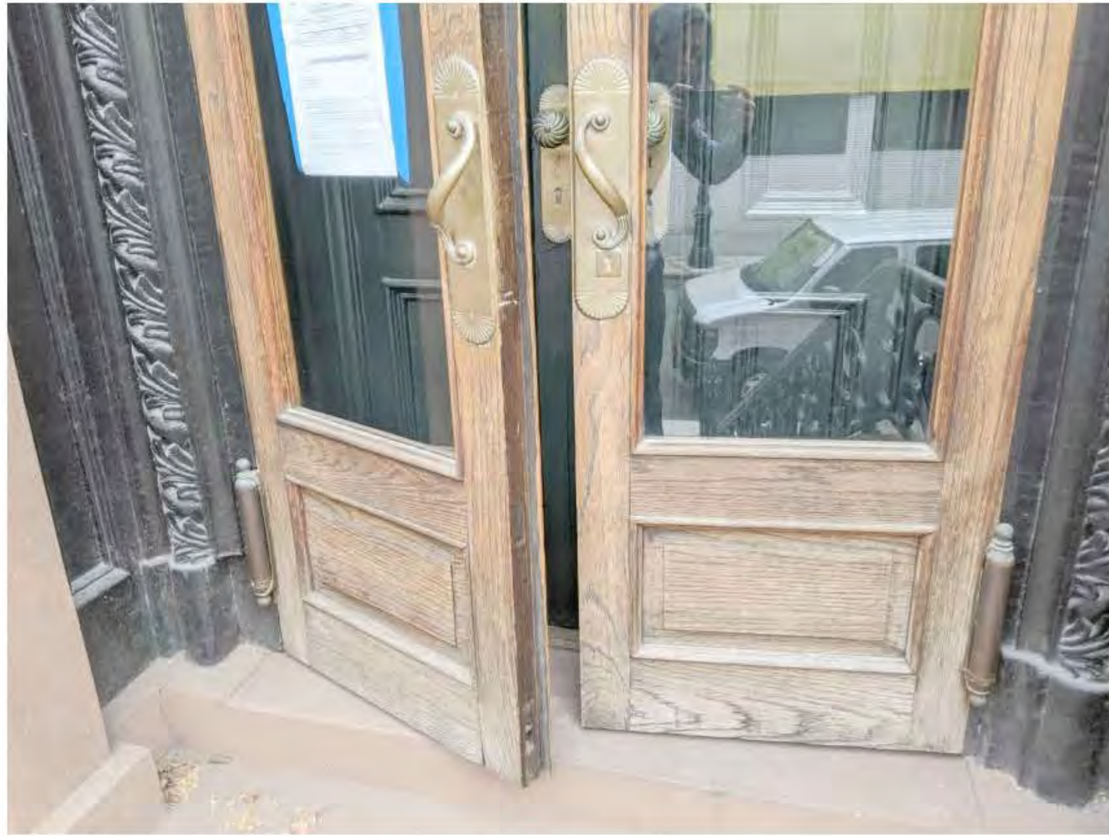
CLOSE UP OF EXISTING ENTRY DOORS (DATE OF PHOTO 03/03/20) NOT TO SCALE
