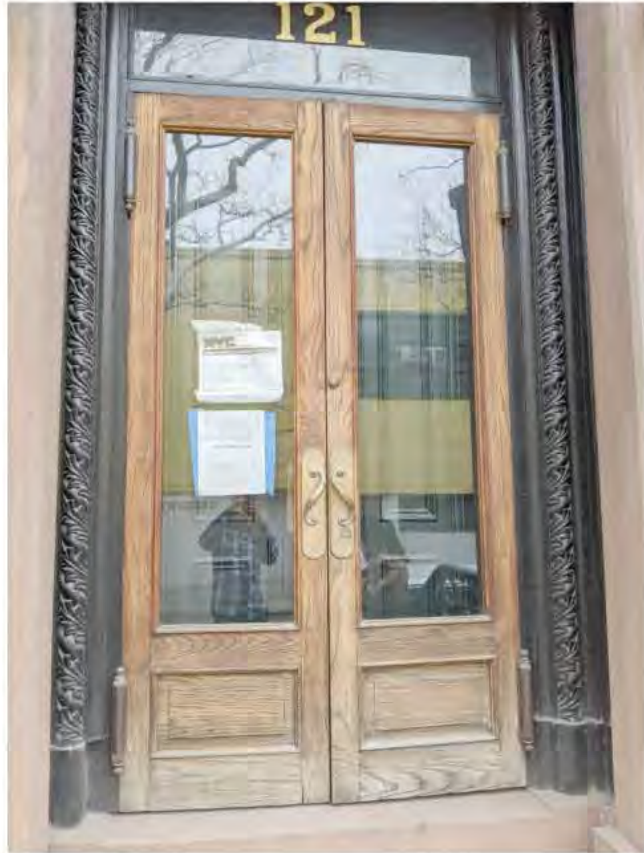
PHOTO OF EXISTING OUTER ENTRY DOORS (DATE OF PHOTO 03/03/20) NOT TO SCALE
