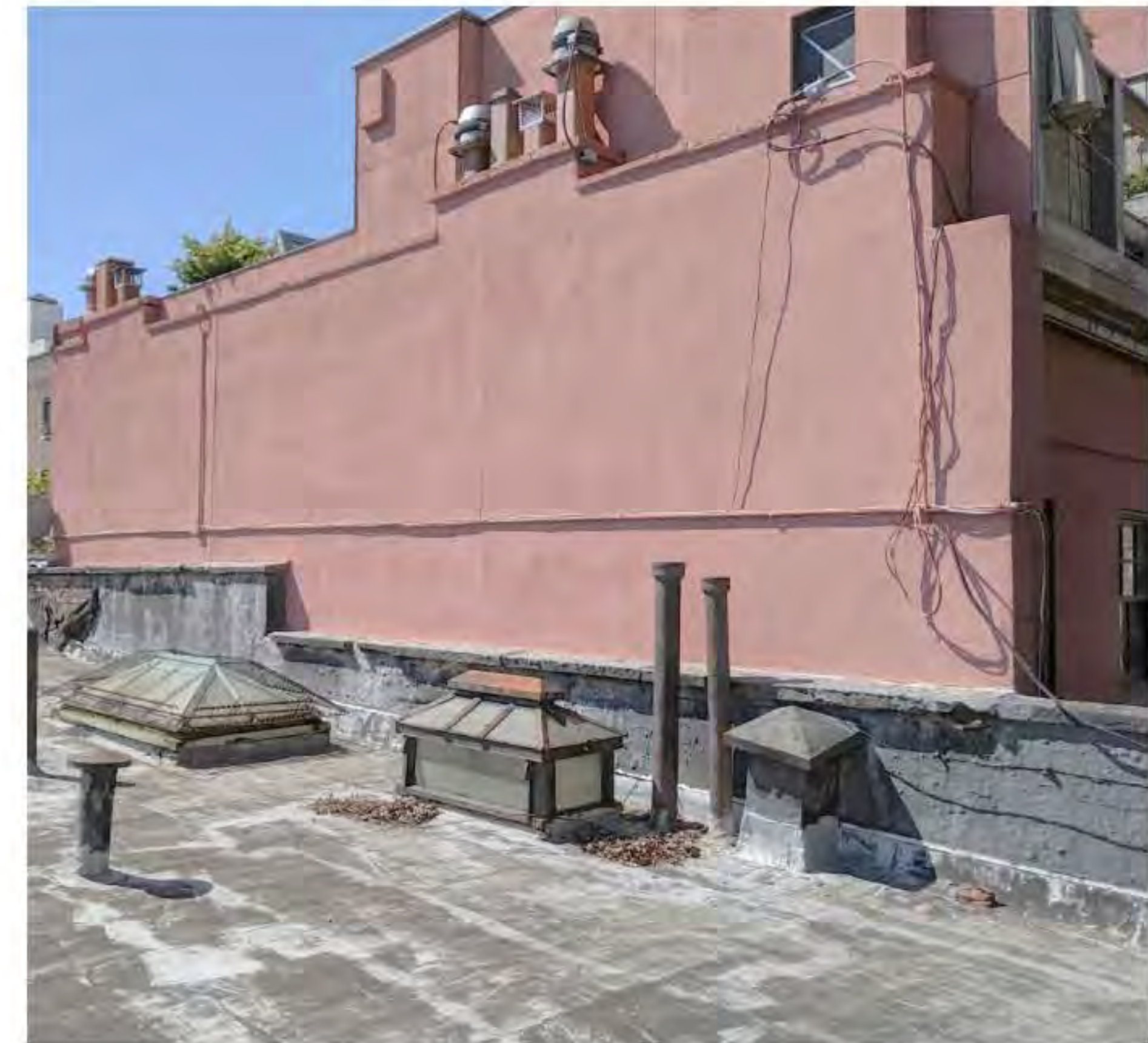
PHOTO OF ROOF - LOOKING WEST 'D' (DATE OF PHOTO 09/17/19) NOT TO SCALE
