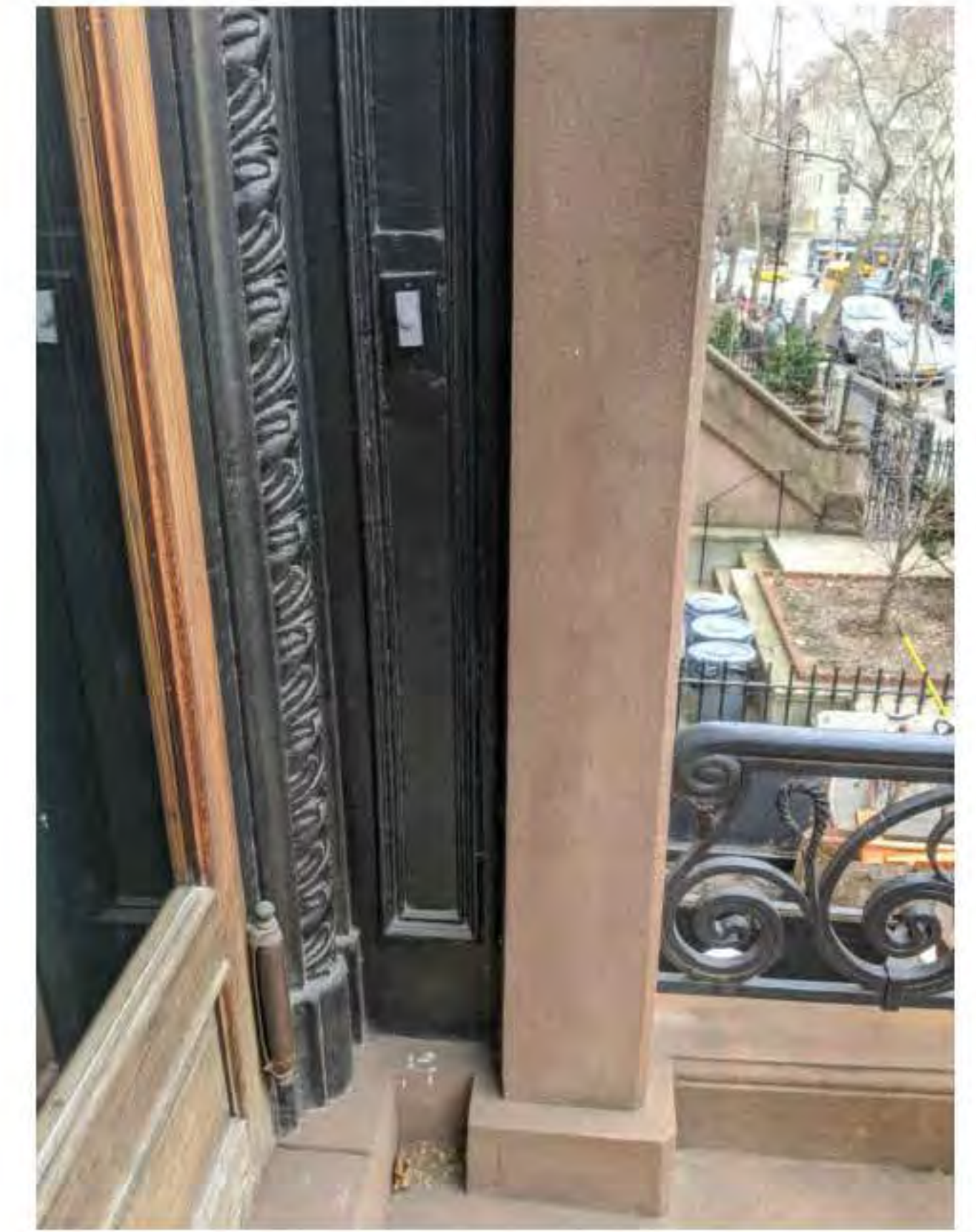
CLOSE UP OF EXISTING ENTRY DOORS LOCATION OF EXISTING DOORBELL (DATE OF PHOTO 03/03/20) NOT TO SCALE
