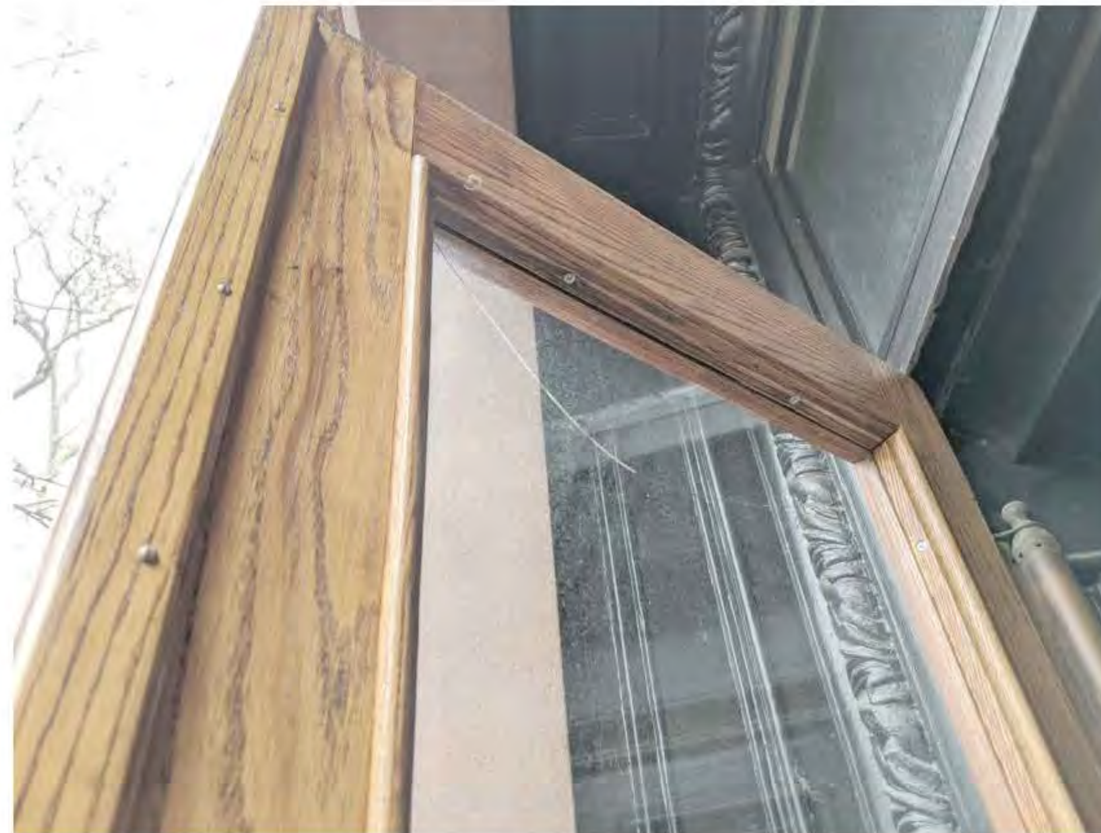
CLOSE UP OF EXISTING ENTRY DOORS BROKEN GLASS IN LEFT OUTER DOOR (DATE OF PHOTO 03/03/20) NOT TO SCALE
