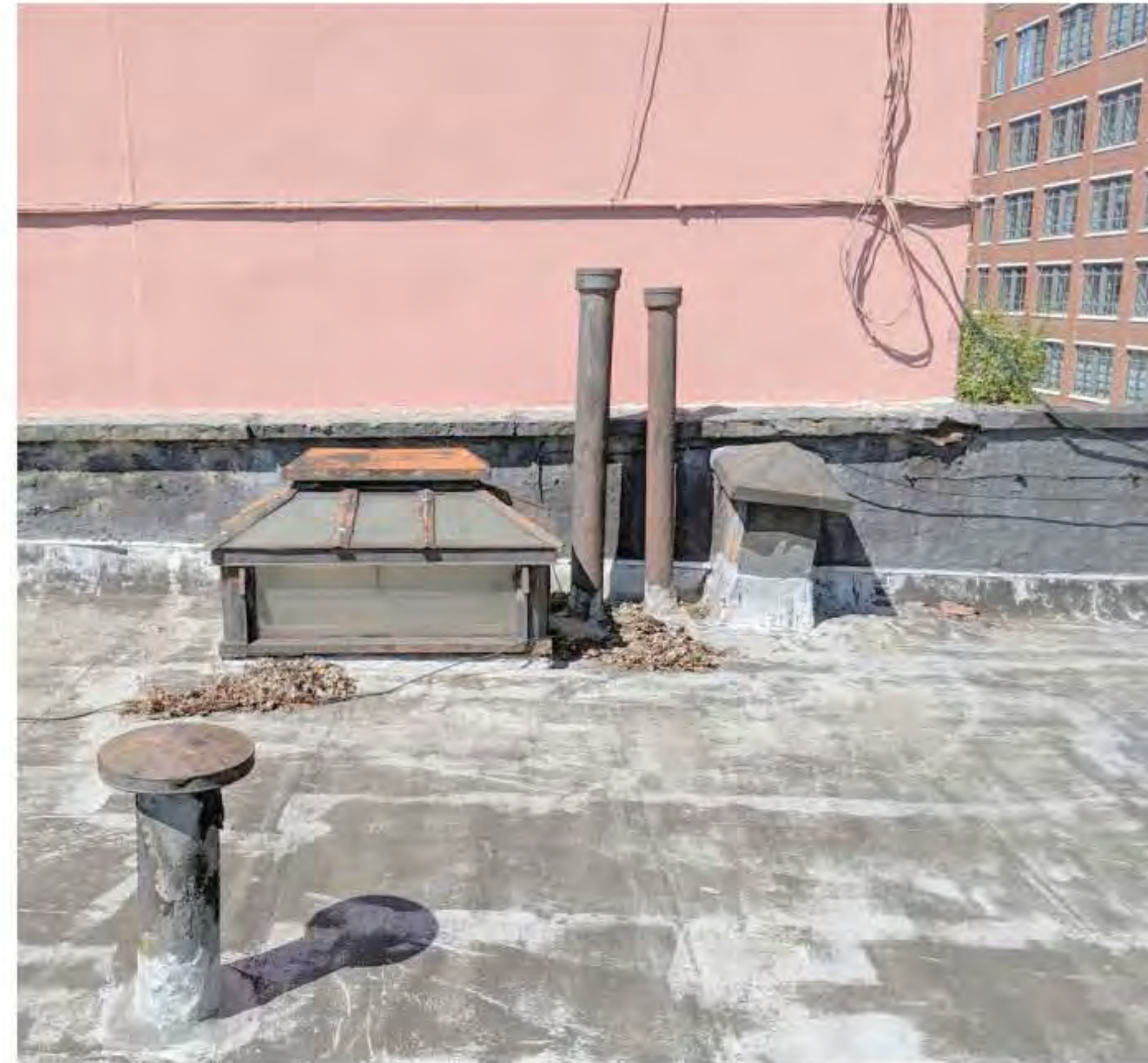
PHOTO OF SKYLIGHTS, FLUES, HATCH AND WEST PARAPET (DATE OF PHOTO 09/17/19) NOT TO SCALE
