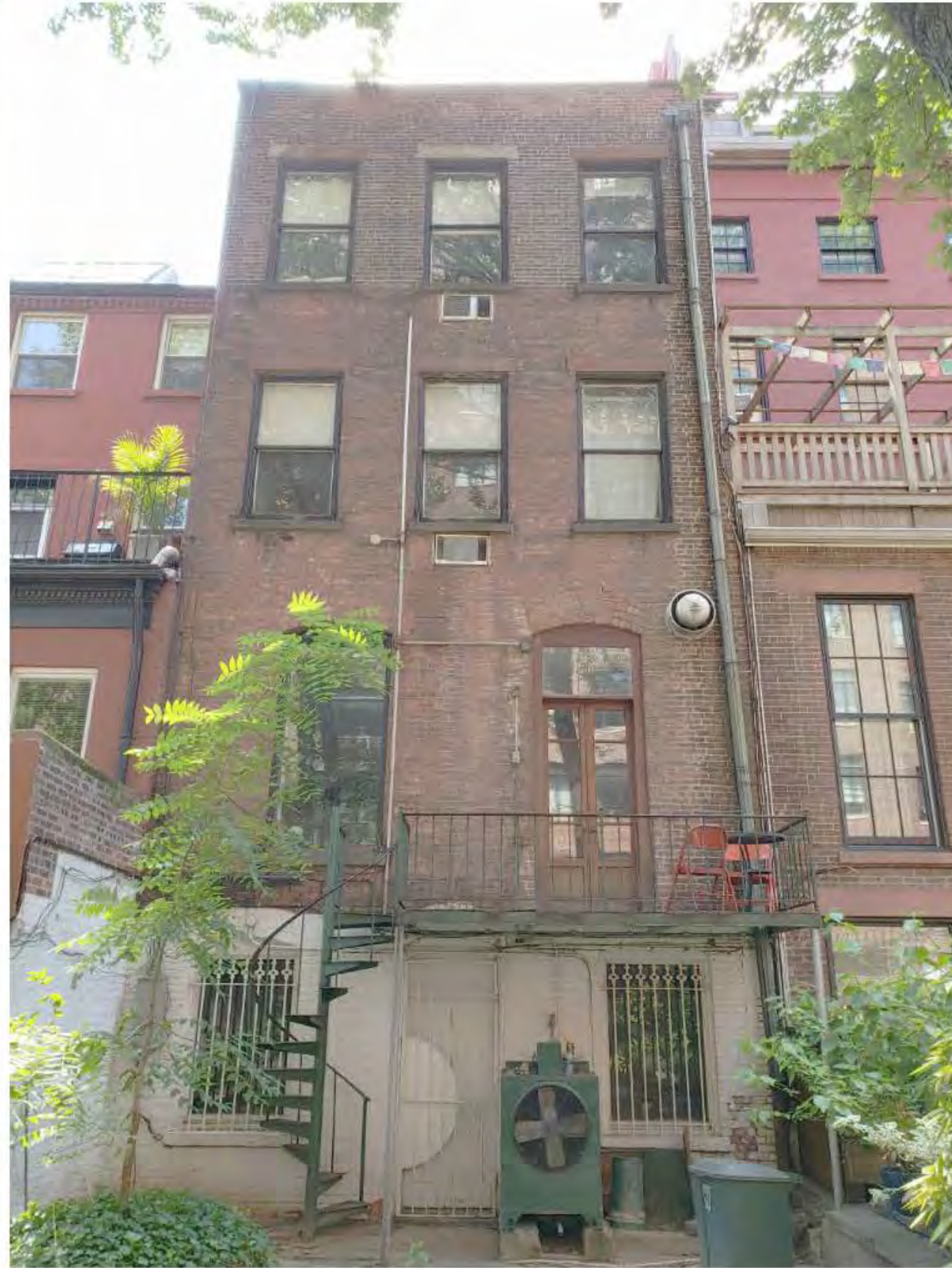
PHOTO OF REAR FACADE - 121 W 11TH ST (DATE OF PHOTO 07/22/19) NOT TO SCALE
